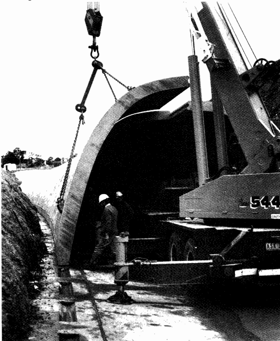
Above: Placing a precast reinforced concrete half arch unit for the Koonung Creek conduit
