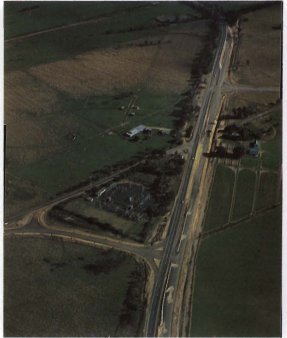
Princes Highway — construction of a staggered 'T' intersection at Racecourse and Army Roads, Pakenham.
