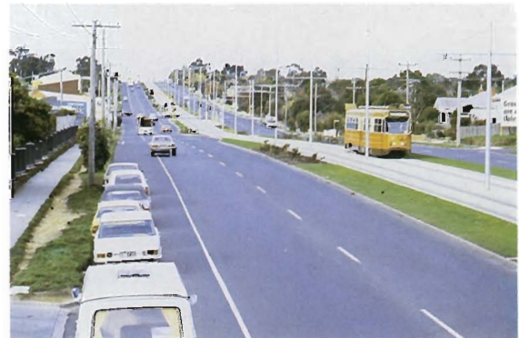
Burwood Highway — completed alterations to highway to allow for extension of tramline from Warrigal Road to Middleborough Road.
