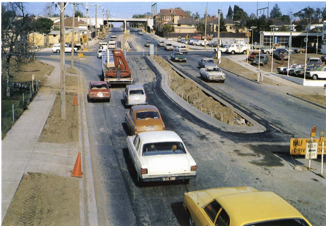
Intersection improvements provide safer roads. Top, Lower Heidelberg Road and Banksia Street, Heidelberg; Below, Maroondah Highway and Elgar Road, Box Hill.
