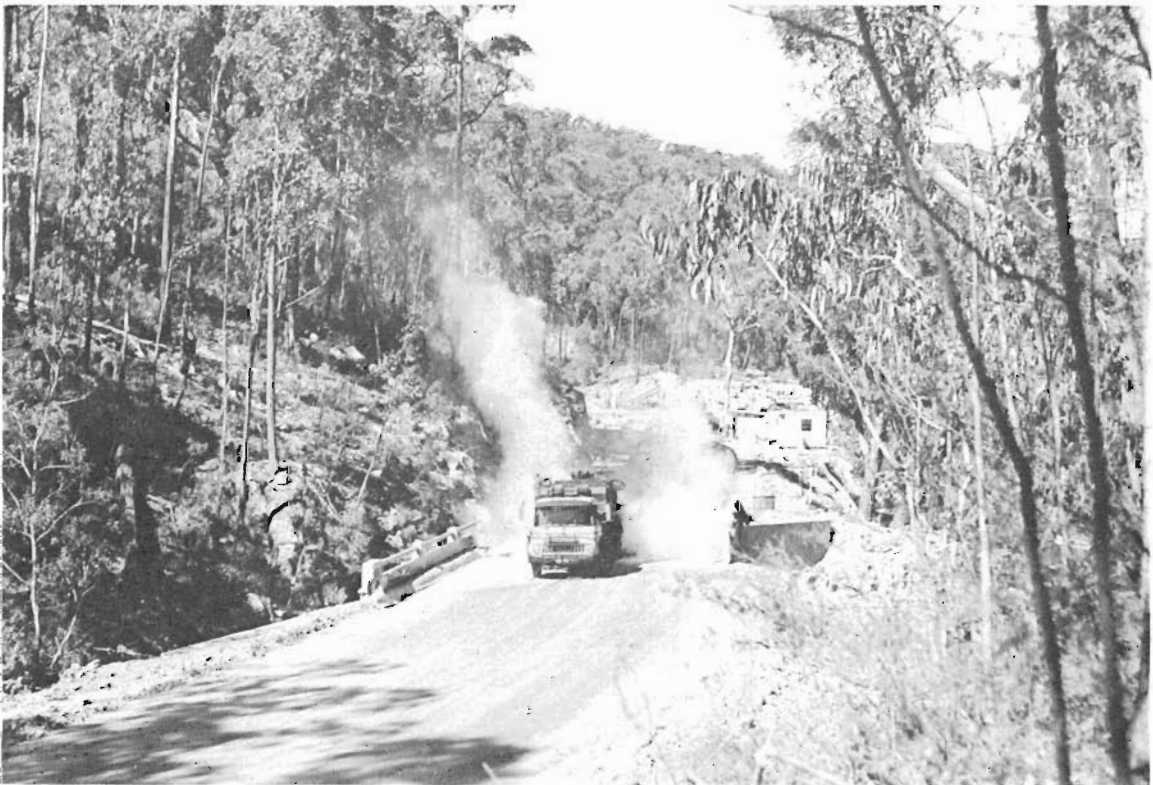
Sealing the deck of the new bridge over Wattle Tree Creek on the Gelantipy Road, Tambo Shire.
