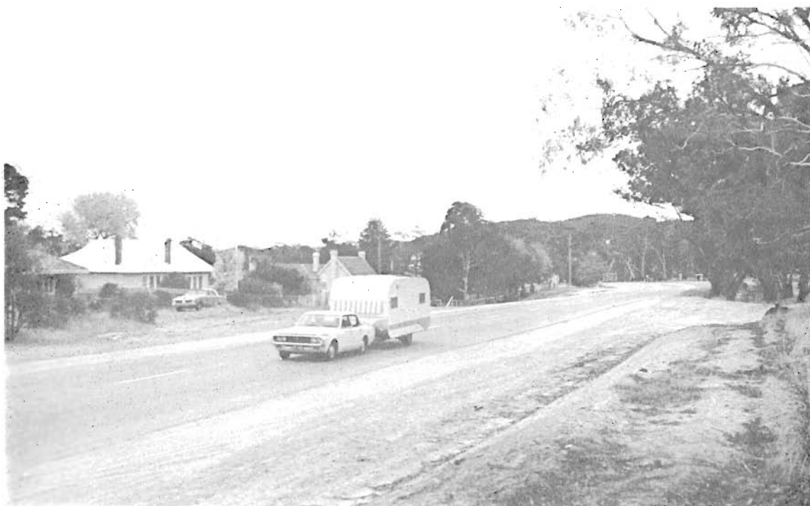
Reconstructed and realigned section of the Goulburn Valley Highway between Trawool and Kerrisdale.
