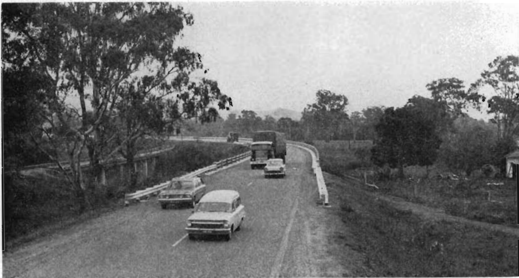
Reconstruction of the Goulburn Valley Highway on a new alignment near Molesworth.
