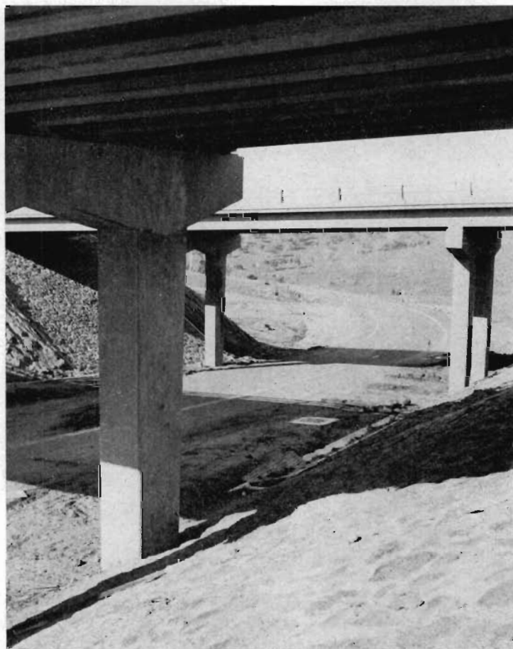
Twin bridges under construction on the Western Freeway (Pentland Hills Section) at the Lion Park interchange.
