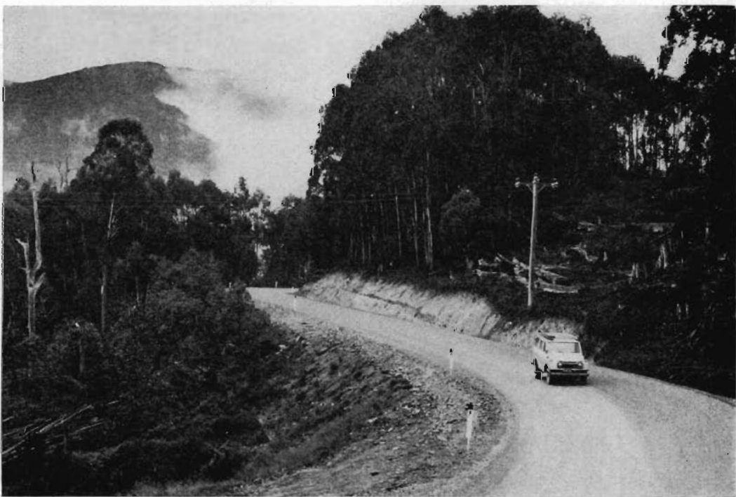
Reconstructed section of the Bogong High Plains Road between Howmans Gap and Falls Creek.
