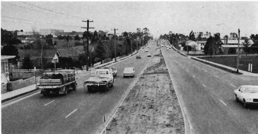
Springvale Road, Waverley City — additional carriageway constructed between High Street Road and Waverley Road.
