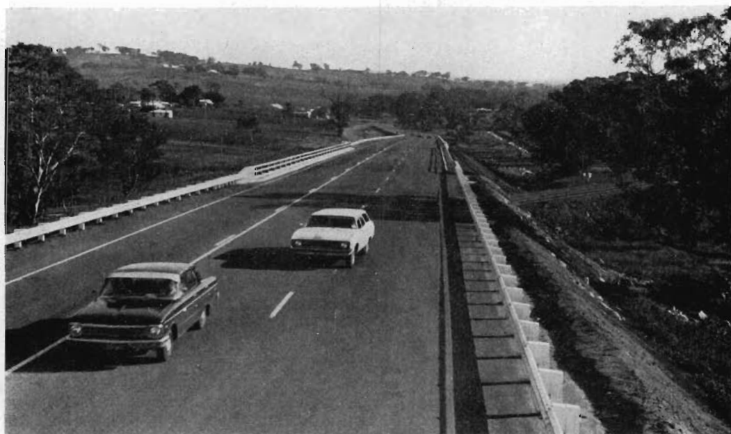
Special Project No. 31 — realignment of the Calder Highway and a new road over rail overpass at Porcupine Hill.
