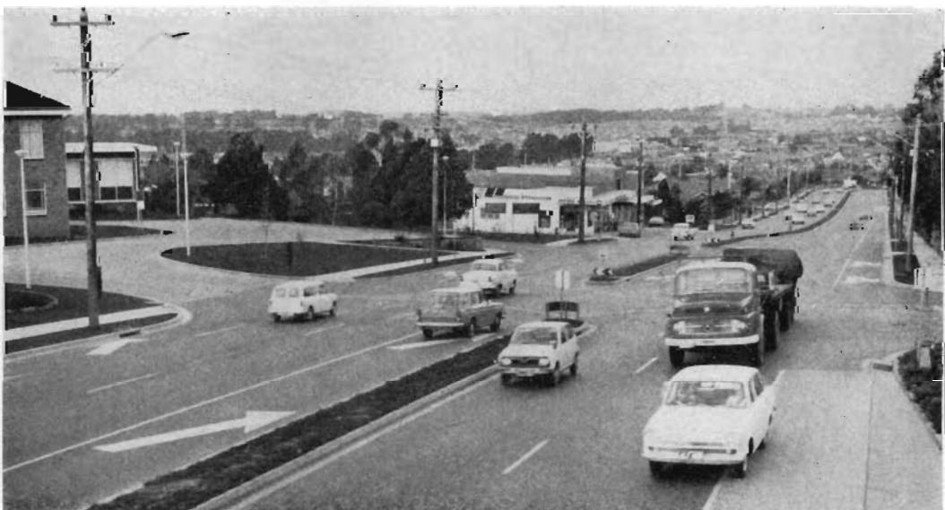
Dual carriageways constructed on Doncaster Road, City of Doncaster and Templestowe City.
