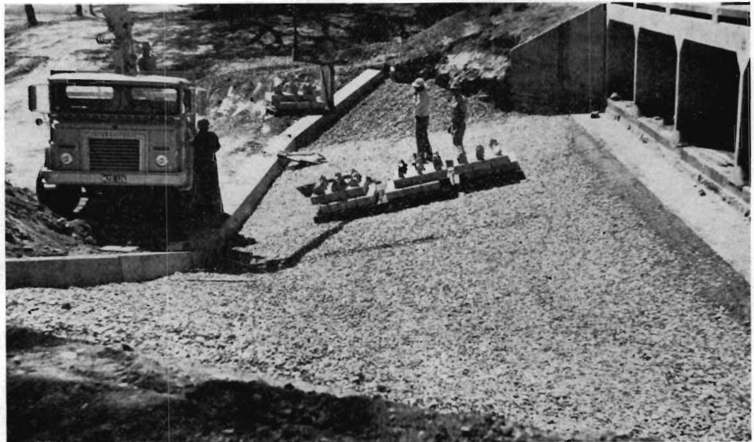
Plate 5—Filter layer spread level with top of upstream cap. The design of the precast concrete dissipator blocks to facilitate interlocking may be seen.
