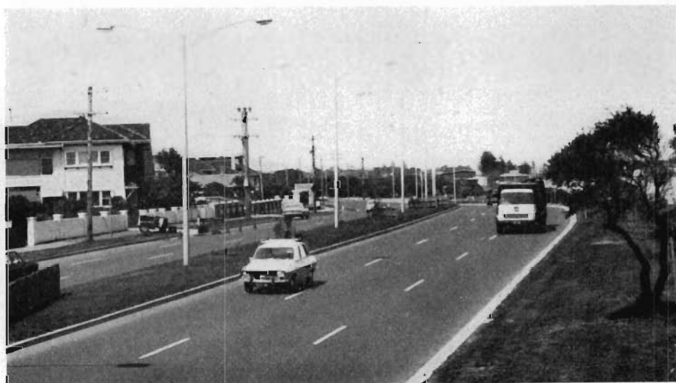
Dual carriageways constructed on Beach Road, north of Normandy Road, City of St. Kilda.
