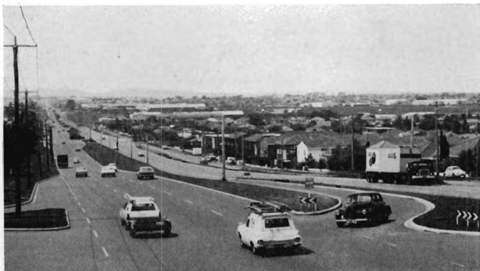
Dual carriageways constructed on Wellington Road east of the Princes Highway, City of Oakleigh.
