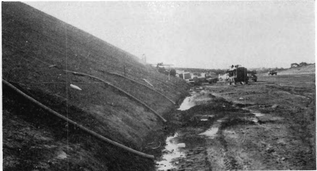
Plate 11—Drilling horizontal sub-surface drains at Mulgrave Freeway. PVC pipe is shown leading from completed drains.
