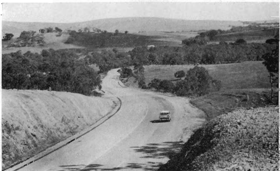
Reconstruction to provide climbing lanes on the Ararat-Halls Gap Road at Copes Hill, Shire of Ararat.
