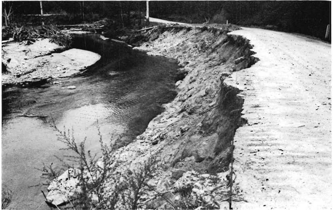
Flood damage to the Cann Valley Highway 16 miles north of Cann River.
