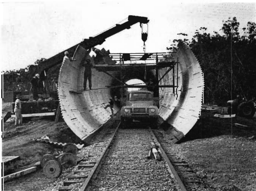
Plate 4—Lyons grade separation structure: placing and bolting of multiplate ring, using a crane and motor truck mounted scaffolds.
