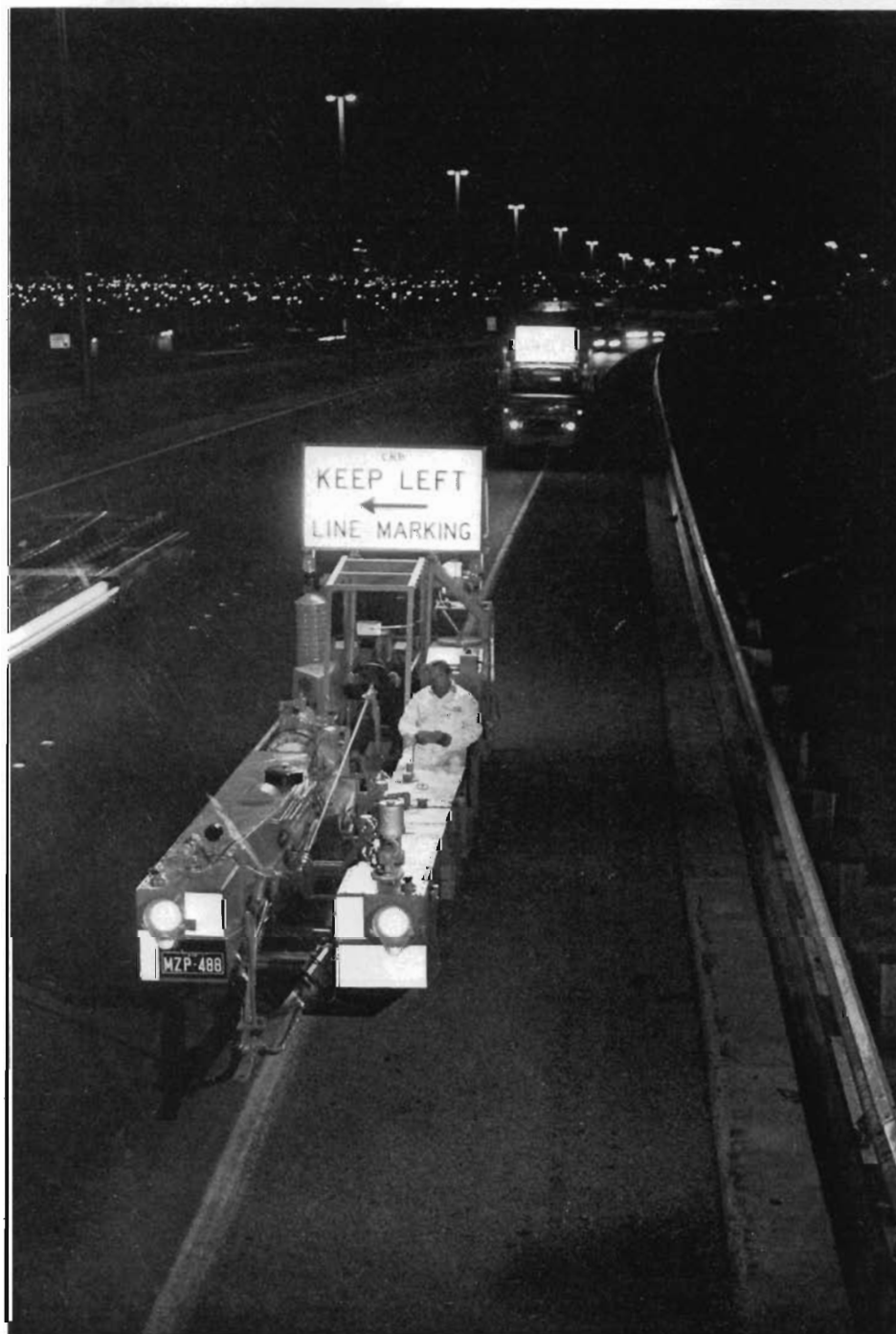
Linemarker on the Lower Yarra Freeway
