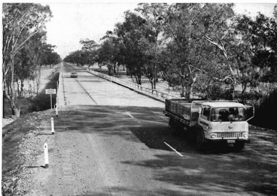
Bridge over Seven Creeks on the Goulburn Valley Highway which was widened to 28 feet between kerbs.
