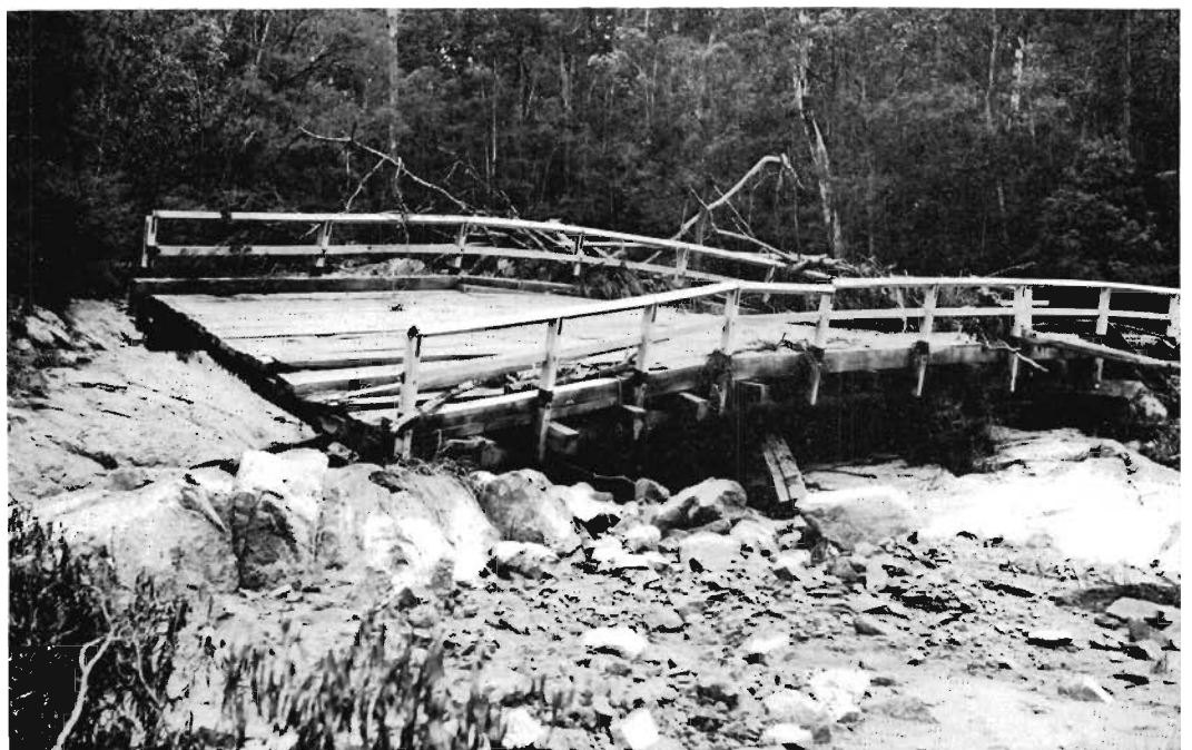
Bridge at Winnets Creek on the Cann Valley Highway damaged by floods.
