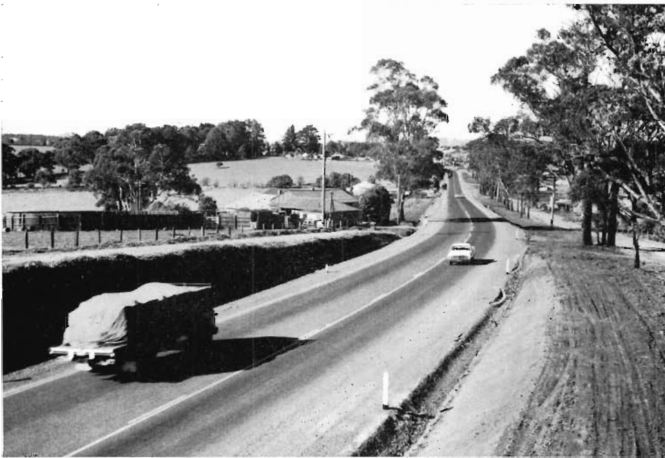
Princes Highway East, Shire of Buln Buln. Reconstruction and realignment between Robin Hood and Drouin.
