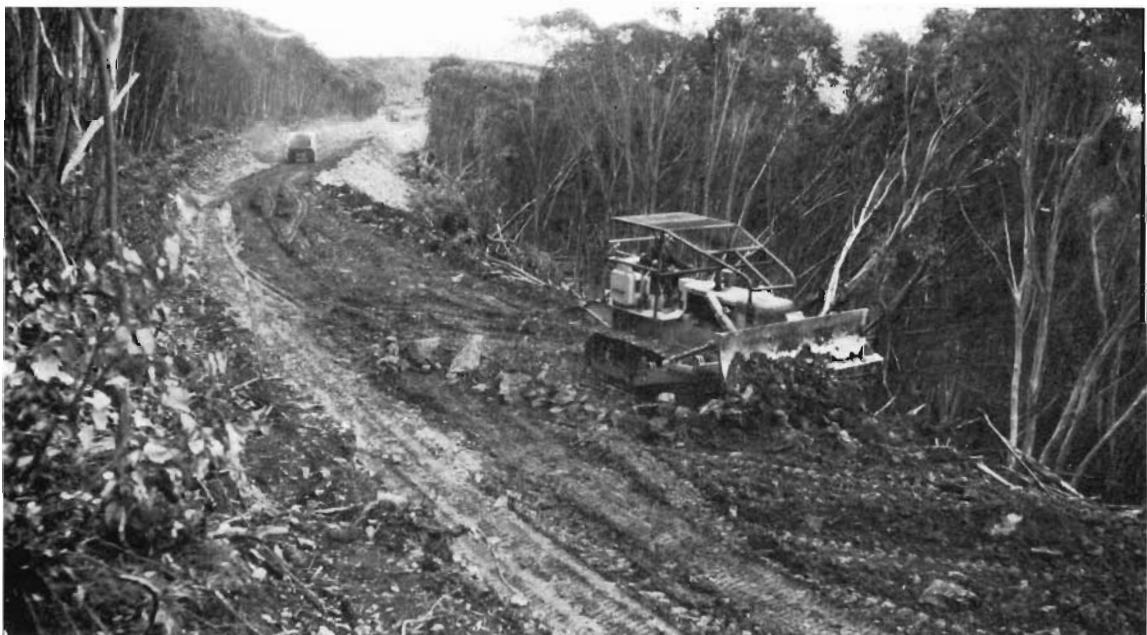
Special Project No. 15. The Jamieson-Licola Road. Construction in progress near Mount Skine.
