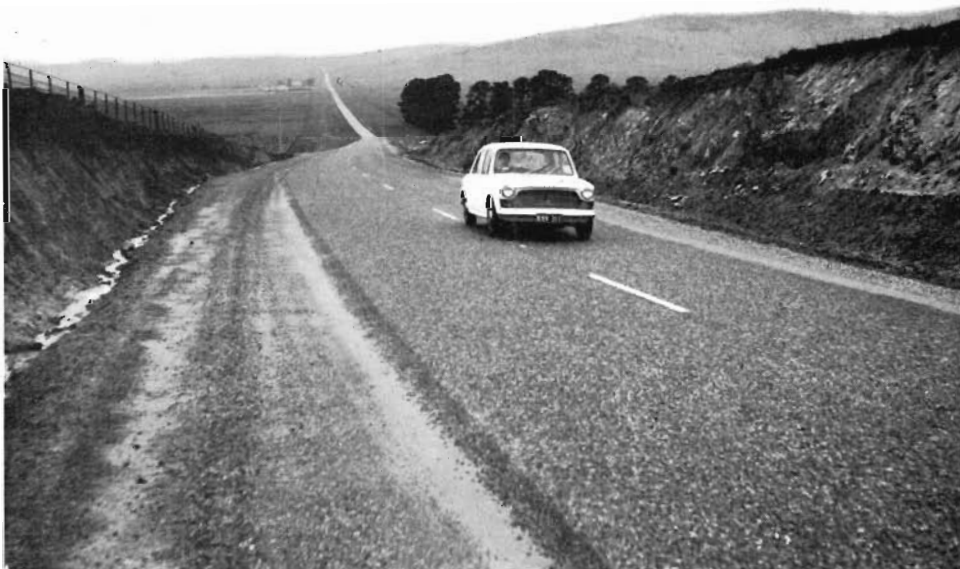
Benambra Road, Shire of Omeo. Reconstruction to provide a sealed pavement 12 feet wide.
