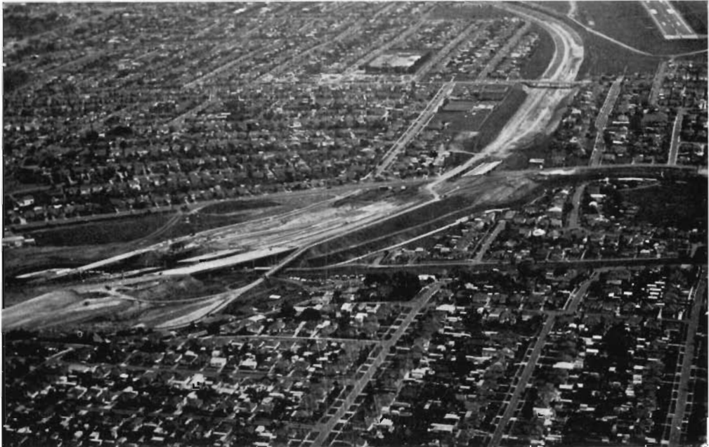
View looking west along the Strathmore By-pass Road under construction, showing the bridge structure.
