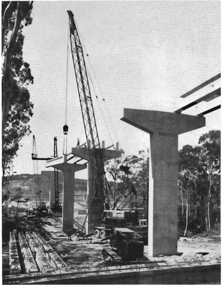
Princes Highway West, Shire of Portland. The Glenelg River Bridge at Dartmoor during construction.
