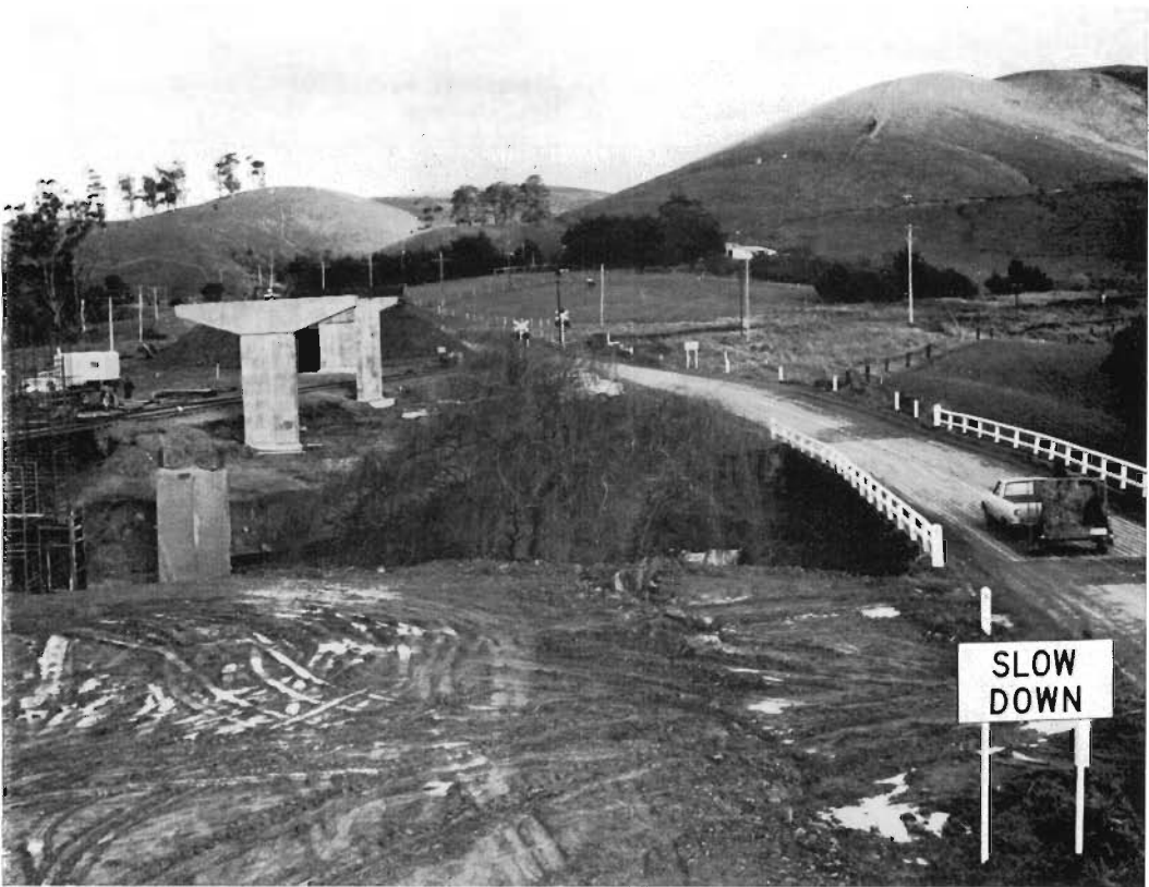
South Gippsland Highway, Shire of Korumburra. Construction of an overpass of the south-eastern railway line and Alsops Creek.
