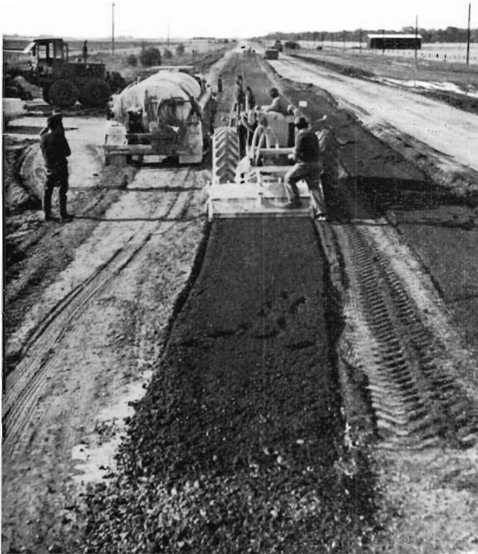
Northern Highway, Shire of Rochester. Reconstruction with lime stabilisation north of Rochester.
