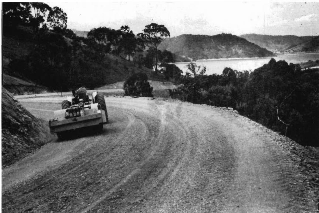
Work is progress on the approach to the Frazer National Park—Lake Eildon in the background.
