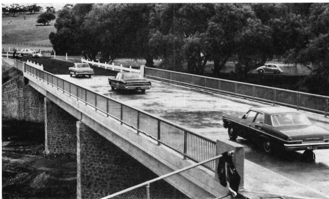
Darley Bridge on Gisborne-Bacchus Marsh Road—Over the Lerderderg River—Shire of Bacchus Marsh.
