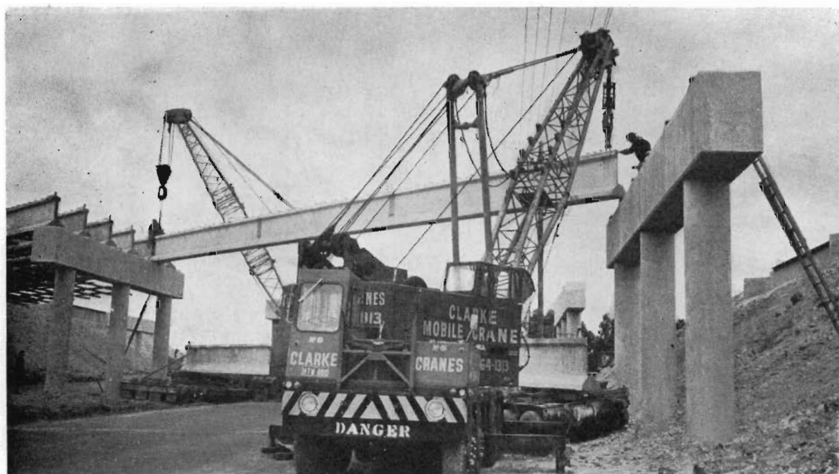
Plate 11.—Dual bridges under construction at the Mickleham Road intersection—Tullamarine Freeway—City of Broadmeadows.
