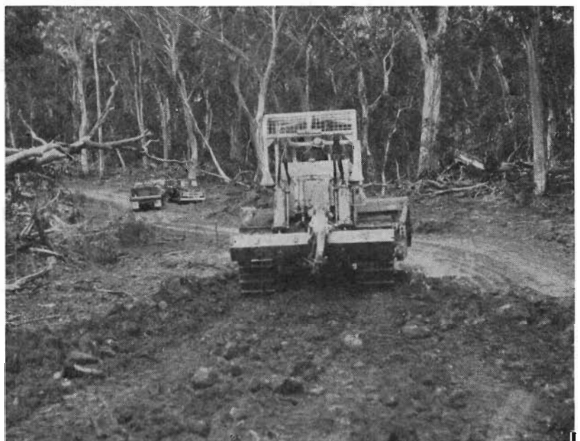
Plate 6.—Omeo Shire—Upper Kiewa Valley Road extension—Construction of a new connecting road from the Rocky Valley Reservoir to the Omeo Highway.
