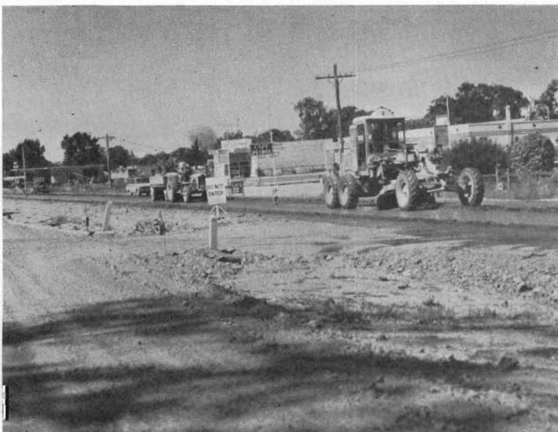
Plate 11.—Hume Highway—Construction of the approaches to the new bridges over the Ovens River at Wangaratta.
