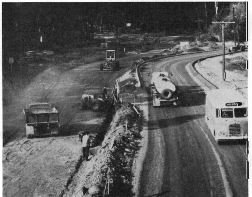
Plate 21.—Burwood Highway— Work in progress at the intersection with Monbulk Road and Mt. Dandenong Tourists' Road.
