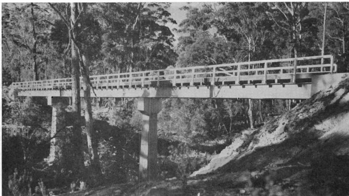
Plate 25.—Shire of Orbost—Combienbar Road—New bridge over the Bemm River at Club Terrace.
