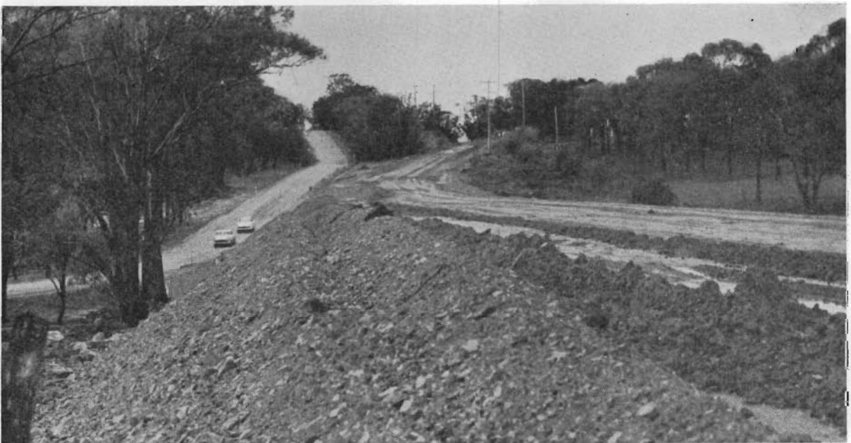
Plate 12.—Hume Highway Section 3. Reconstruction in progress north of Winton. Shire of Benalla.
