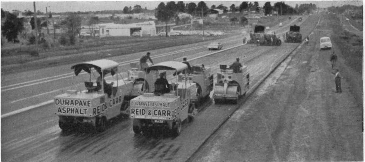
Plate 1.—Princes Highway East Section I.—36 ft. wide hot mix seal being laid east of Springvale Road. City of Springvale.
