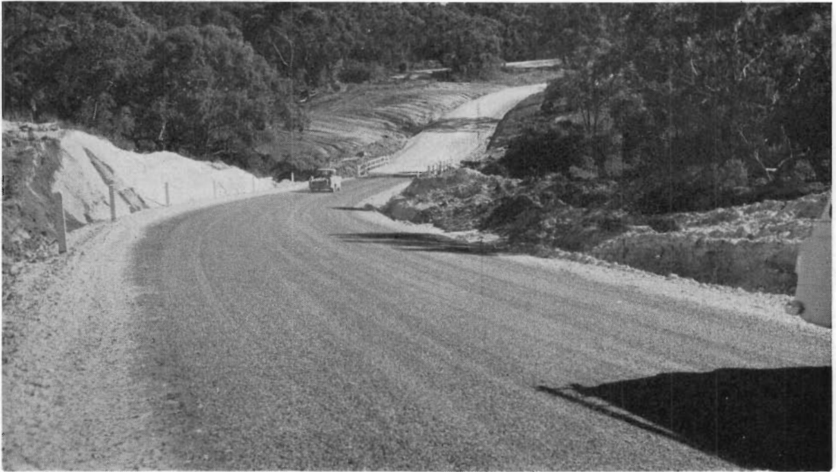
Plate 36.—Portland Shire. Drik Drik—Nelson Road. Reconstructed and sealed section south of Drik Drik.
