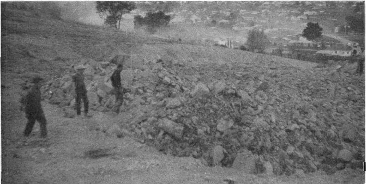
Plate 2.—View of upper end of section after firing, showing comparatively larger size stone at end of section and small amount of stone thrown onto batter.
