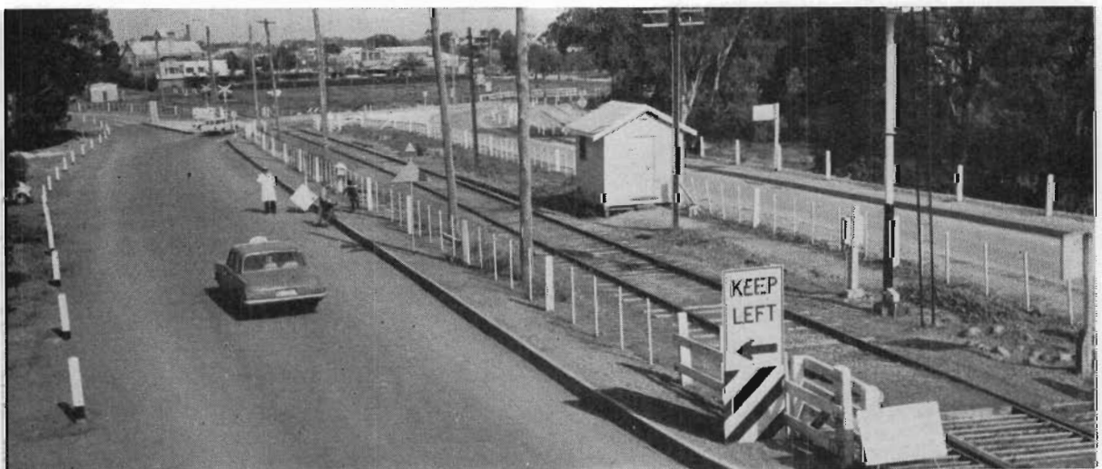
Plate 51.—Department of Public Works. Northern Highway—Realignment at fruit fly inspection point near Murray River Bridge—Echuca.
