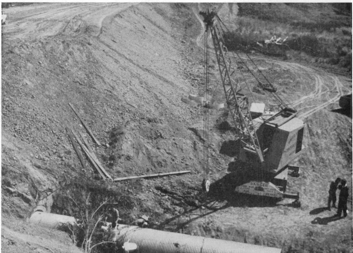
Plate 15.—South Gippsland Highway. Installing armco pipe in old railway embankment immediately east of Korumburra.
