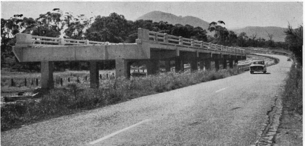
Plate 43 and 44.—Maroondah Highway. Two of the series of bridges over Yarra Flats, near Healesville, to raise pavement above flood level.
