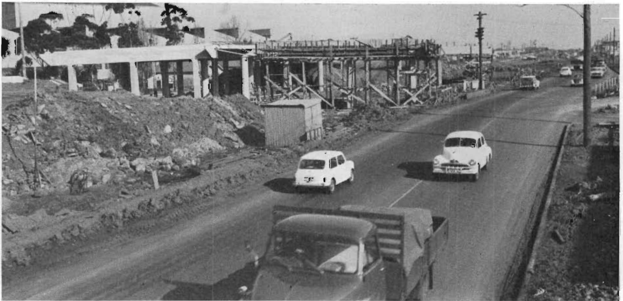
Plate 5.—Princes Highway West Section I.—Construction of railway overpass at Brooklyn. City of Sunshine.
