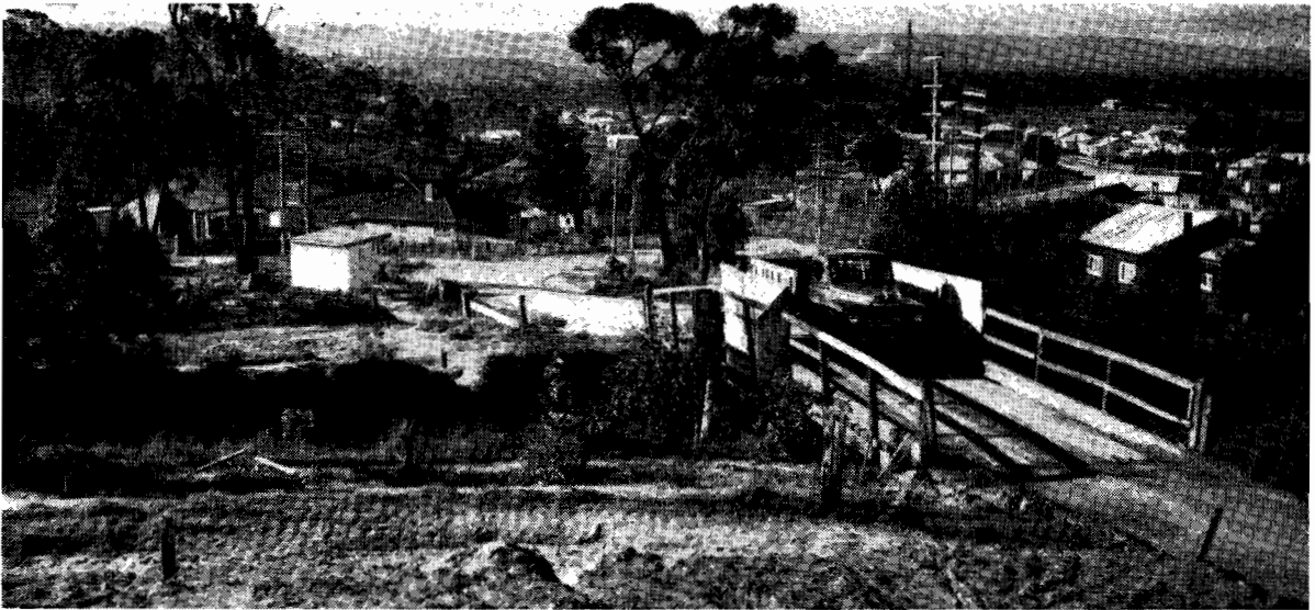
Plate 2.—Princes Highway East. Site of new crossing over railway on deviation at Hernes Oak prior to construction.
