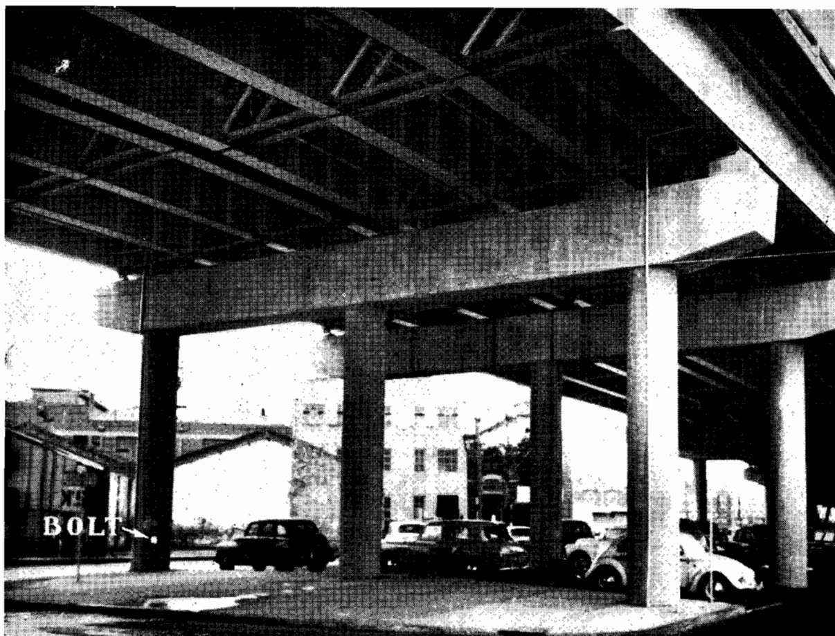
Plate 7.—Kings Bridge, showing typical position of stainless steel bolt in pier column.
