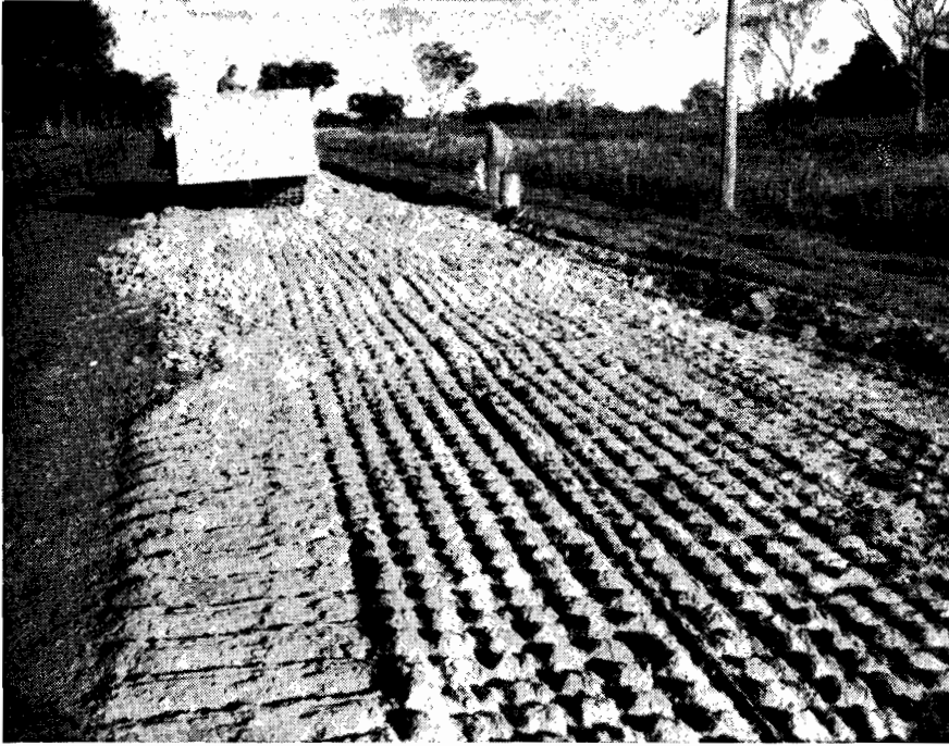
Plate 2.—Grid roller used in raising pavement above flood level, Midland Highway, Section 3.
