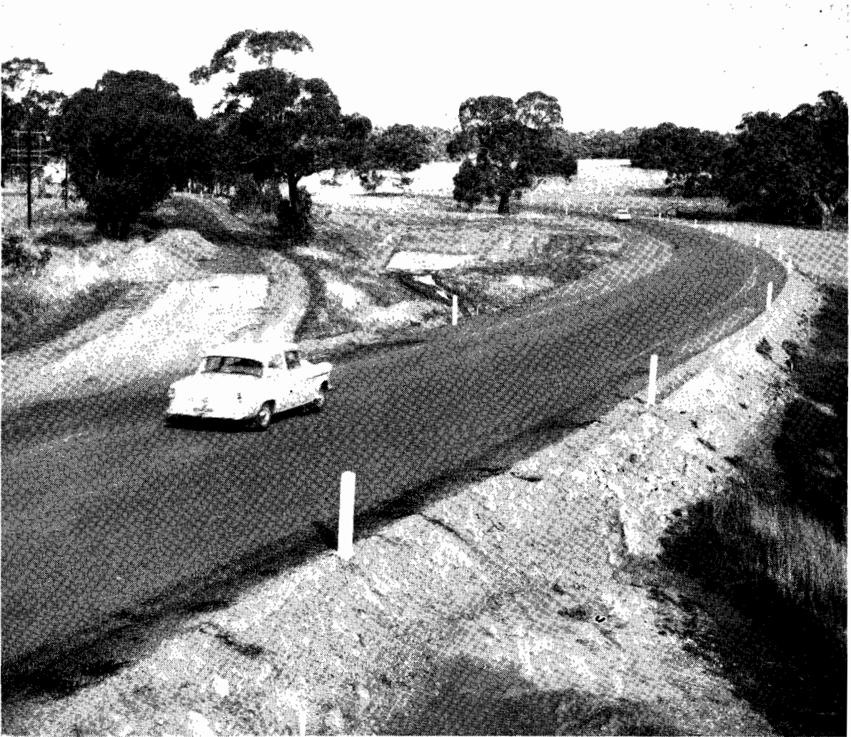
Plate 22.—Shire of Ararat. Ararat-Warrnambool Road. Reconstructed, realigned, and sealed section, south of Ararat.
