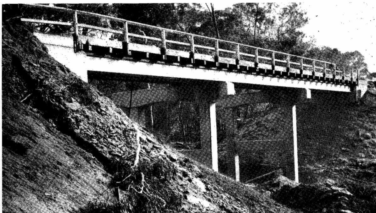
Plate 27.—Shire of Portland. Dartmoor—Hamilton Road. New bridge under construction over Crawford River.
