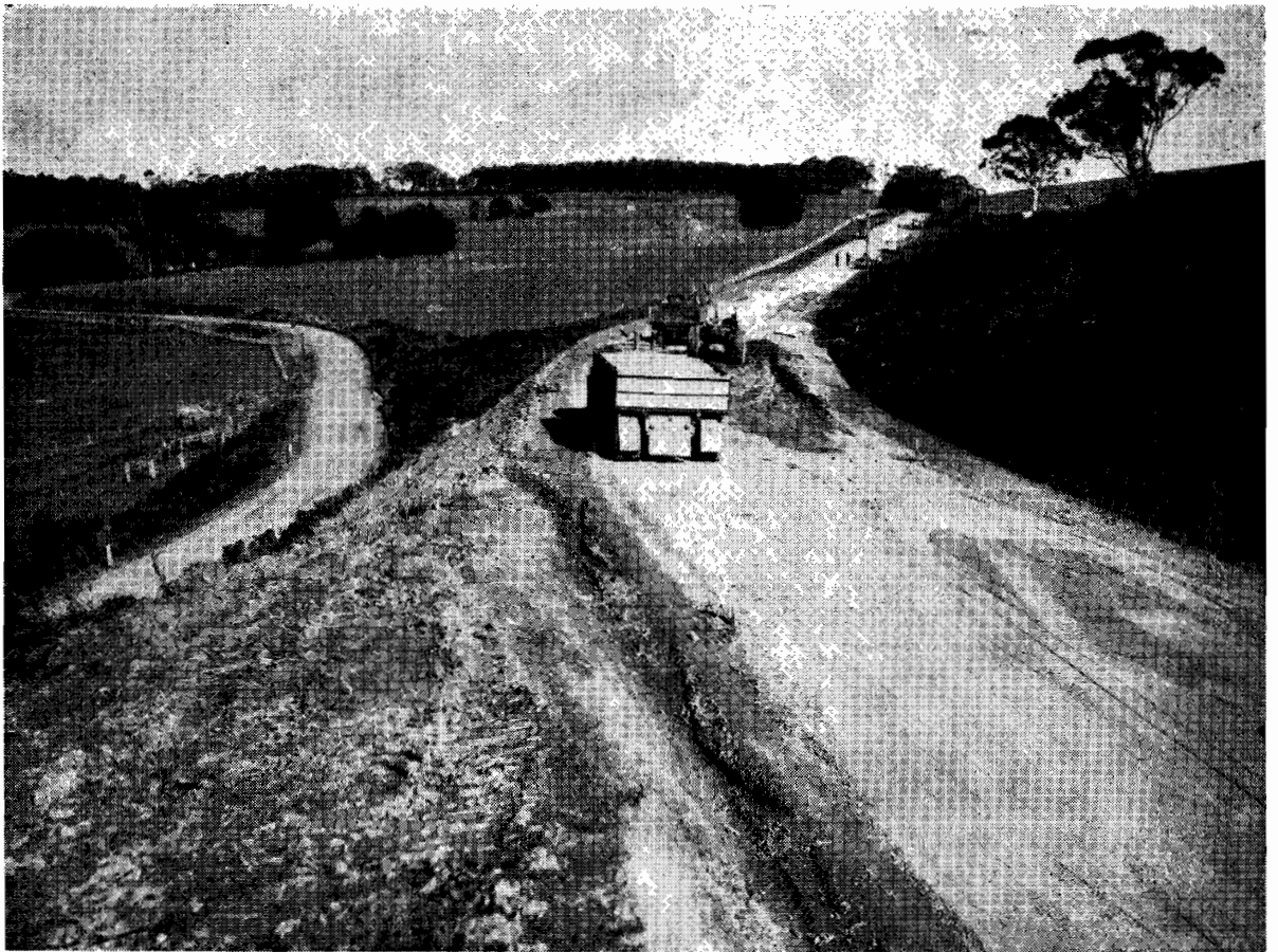
Plate 33.—Shire of Narracan. Walhalla Road. Deviation of road around Moondarra Reservoir. Old road on lower left.
