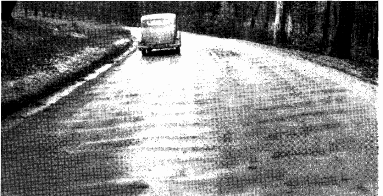
Plate 1.—Before reconstruction (see below) corrugated and pot-holed surface of Tallangatta–Corryong Road, Shire of Upper Murray.
