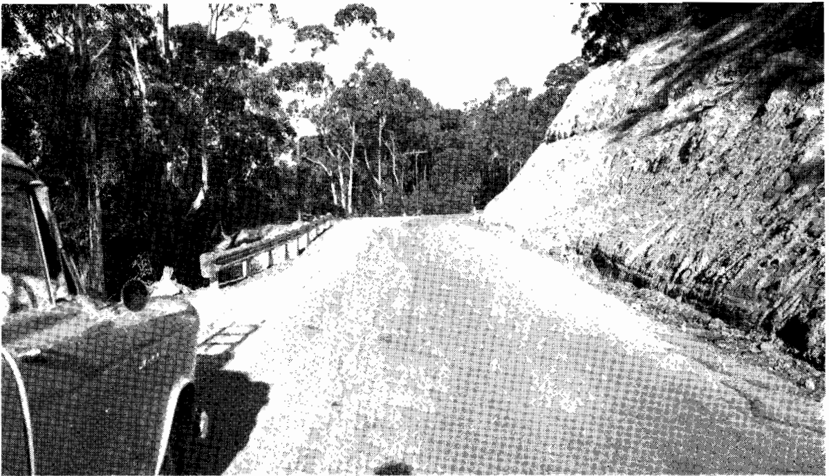
Plate 11.—Ocean Road. Shire of Otway, west of Moonlight Head turn-off after reconstruction and widening.
