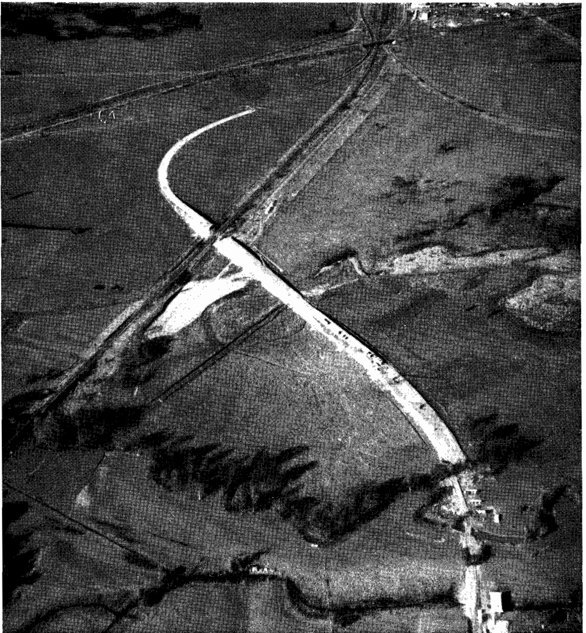
Plate 44.—Princes Highway East. Realignment under construction between Herne's Oak and Morwell, looking towards Morwell.
