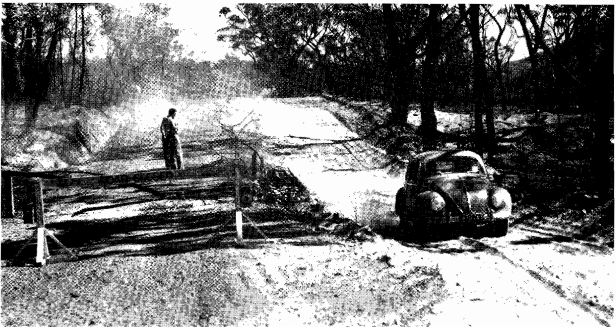
Plate 12.—Shire of Ararat. Grampians Road near Jimmy's Creek. Side track around a timber culvert burnt out by bush fire.
