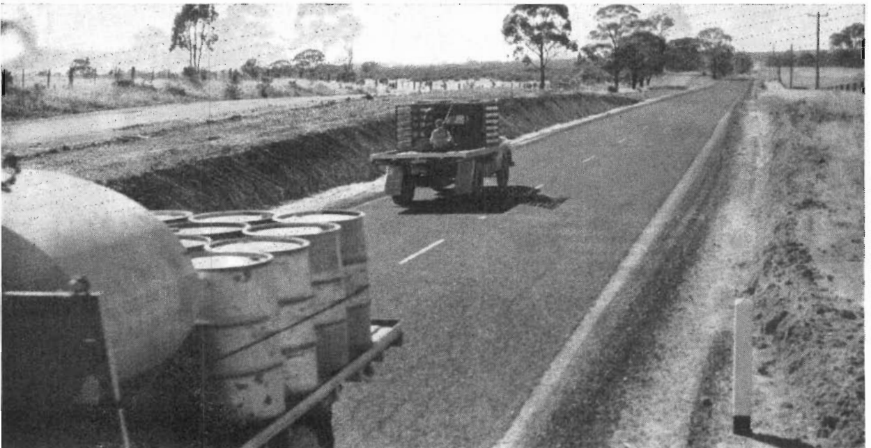
Plate 24.—Midland Highway. Reconstruction between Huntly and Bagshot alongside old worn-out "switch back" section
