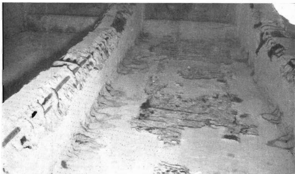
Plate 7.—Fire damage to reinforced concrete bridge on the Hume Highway at Springhurst.
