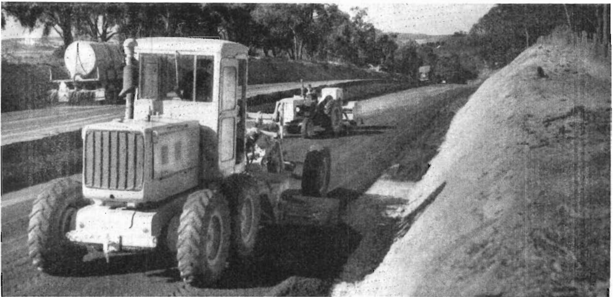
Plate 21.—Hume Highway. Provision of a Climbing lane on Pretty Sally Hill, north of Wallan
