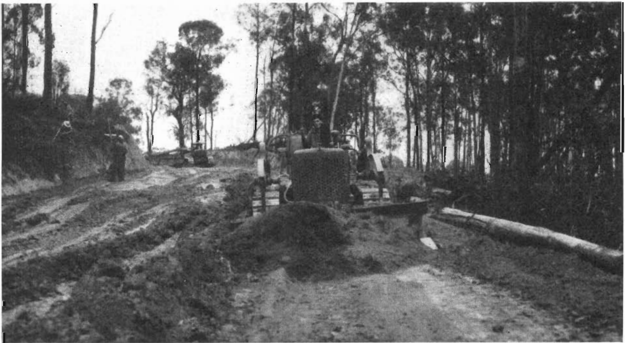
Plate 9.—Shire of Bairnsdale.—Bullamwaal Main Road approximately 7\frac{1}{2} miles from Bairnsdale. Reconstruction in progress.
