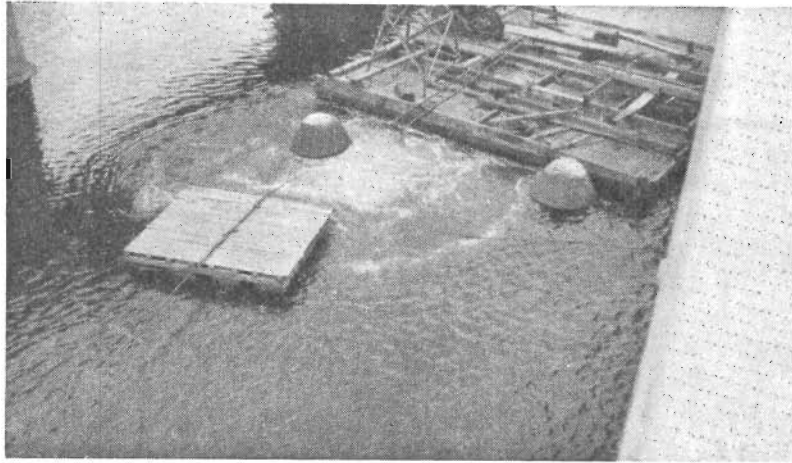
Plate 5.—Underwater Demolition—Bridge over Mitchell River at Bairnsdale. (Note ring of air bubbles.)
