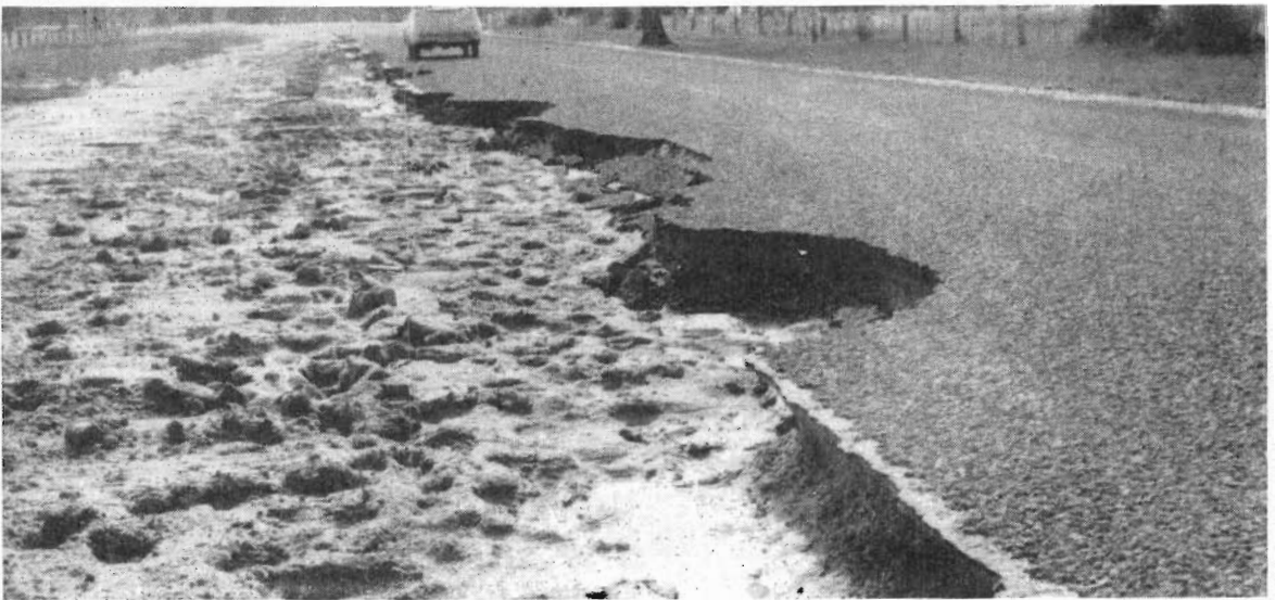
Plate No. 17 :—Murray Valley Highway—Badly damaged, sealed section, after flooding by Goulburn River—Approximately 3 miles south of Nathalia.
