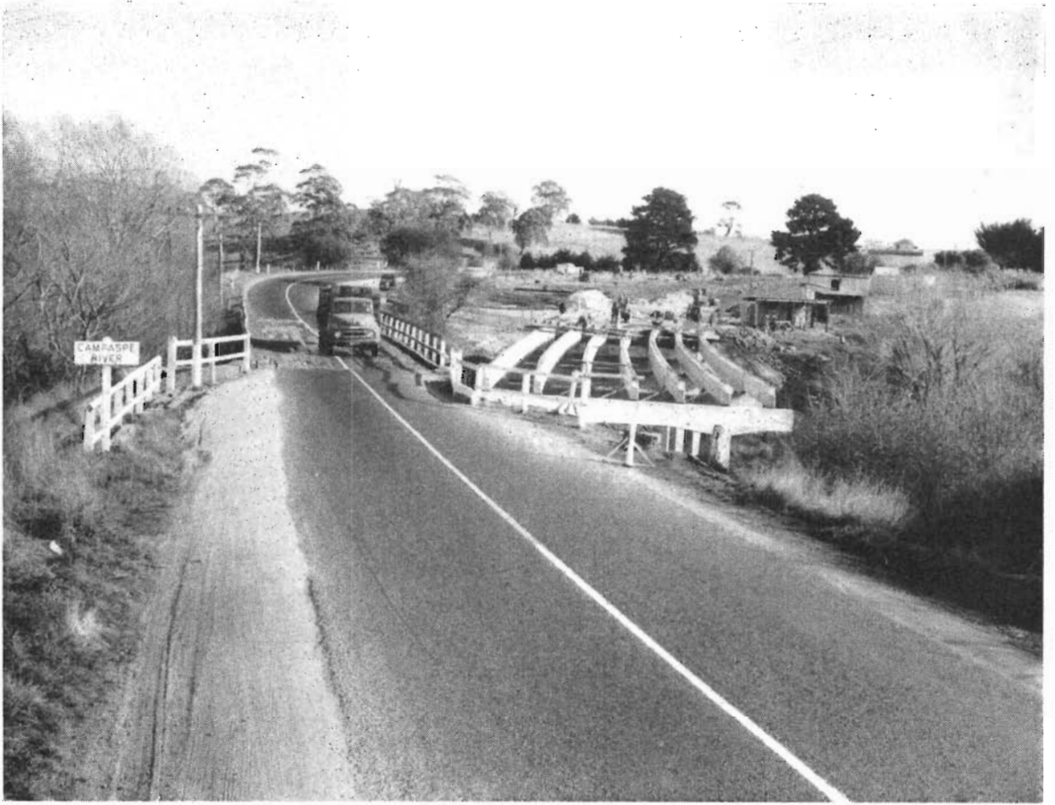
Plate No. 8 :—Calder Highway—Shamrock Bridge over Campaspe River west of Karlsruhe, using precast beams.
