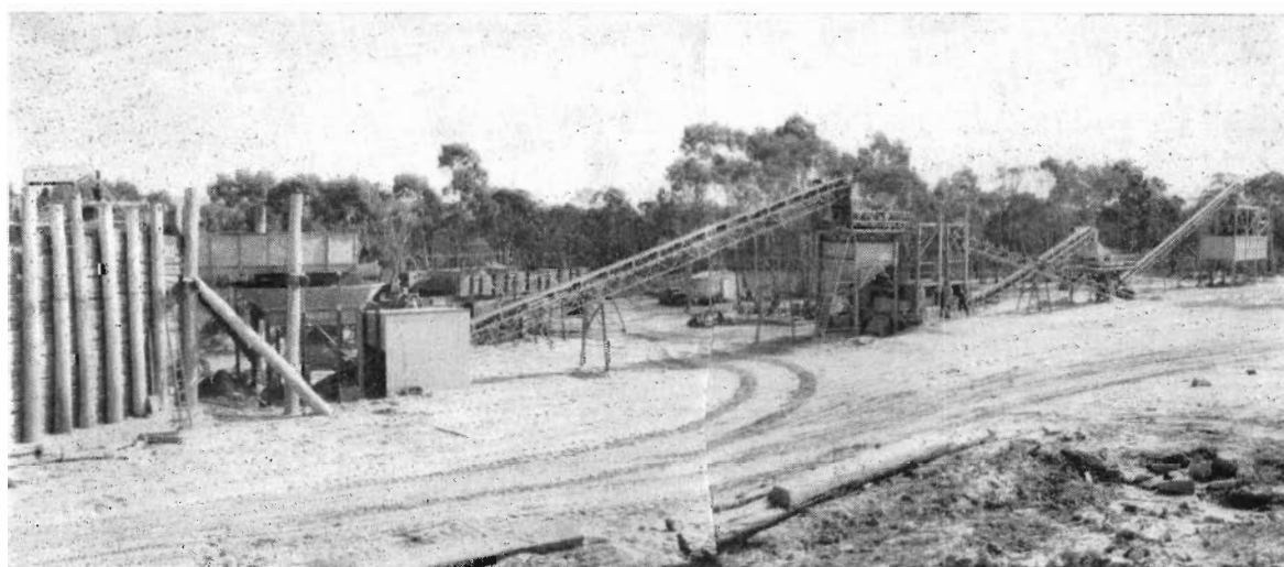
Plate No. 23 :—New plant and screens—Stawell Quarry—Vibrating feeder, elevators, and secondary crushers.
