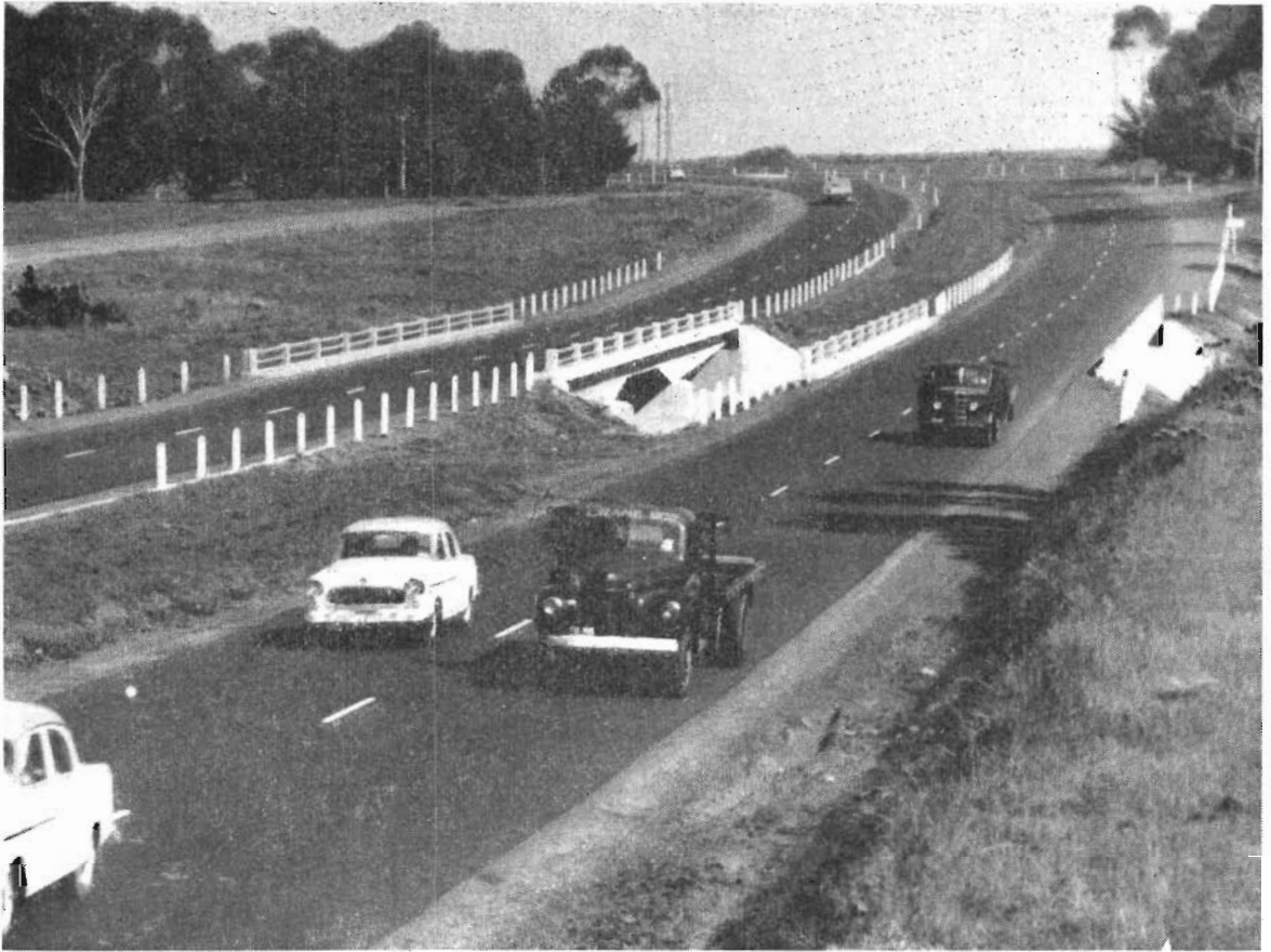
Plate No. 6 :—Princes Highway West at Kororoit Creek—Duplication of pavement and new bridges on new alignment.
