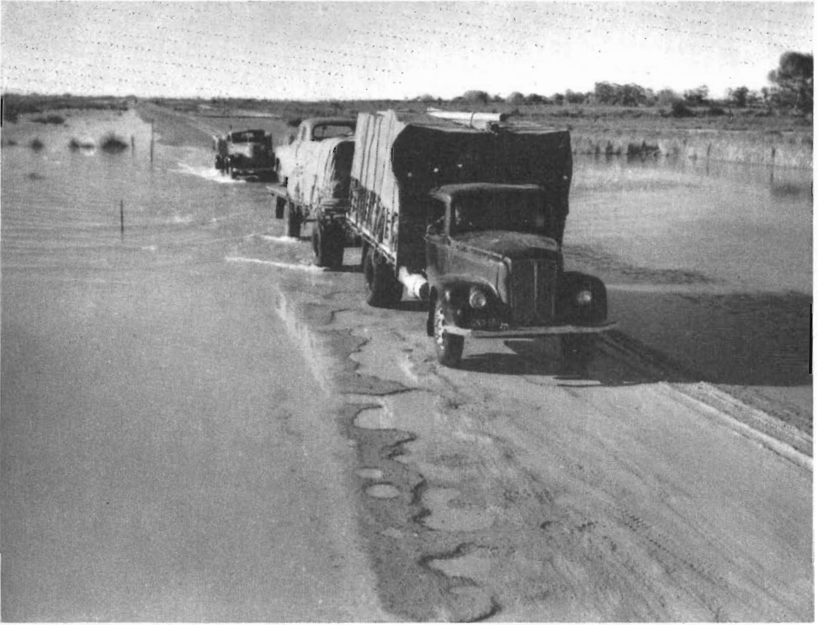
Plate No. 15 :—Murray Valley Highway—Flooded section approximately 2 miles east of Lake Boga showing failed pavement.
