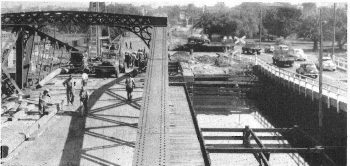
Plate No. 14 :—Cities of Footscray and Melbourne Bridge over Maribyrnong River at Napier Street—Under construction.
