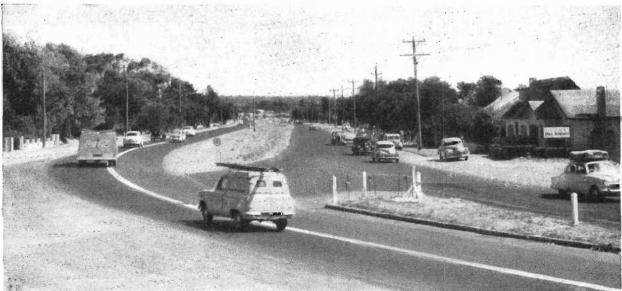
Plate 14.—Nepean Highway. Duplication between Frankston and Mile Bridge. View at Seaford Road intersection—new carriageway on right.
