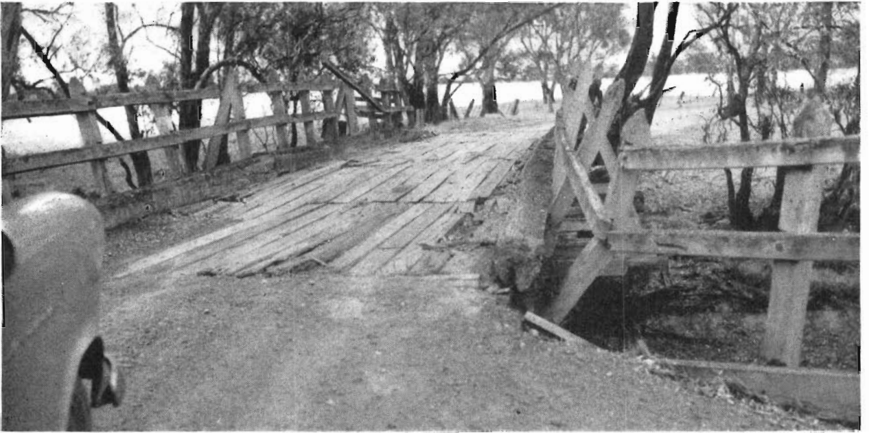
Plate 1.—Old bridge on Murchison-Violet Town Main Road. Loads limited to 6 tons gross. Replacement delayed by lack of funds.
