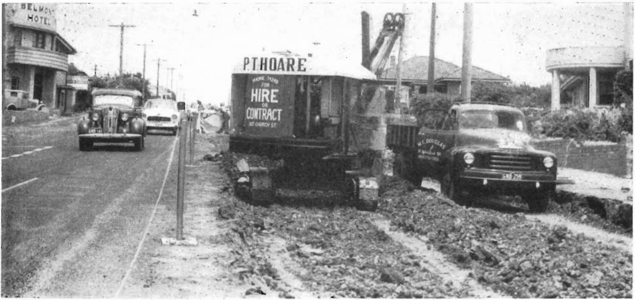
Plate 10.—Reconstruction of Princes Highway West in Belmont to new levels after removal of tramline.
