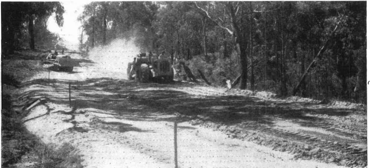
Plates 4 and 5.—Heavy equipment on reconstruction of hilly section of Yarram-Traralgon Road near Carrajung Lower—Alberton Shire.
