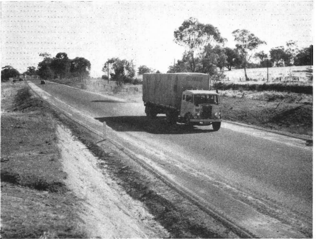
Plate 25.—Hume Highway. New deviation through Glenrowan which eliminates two railway level crossings.
