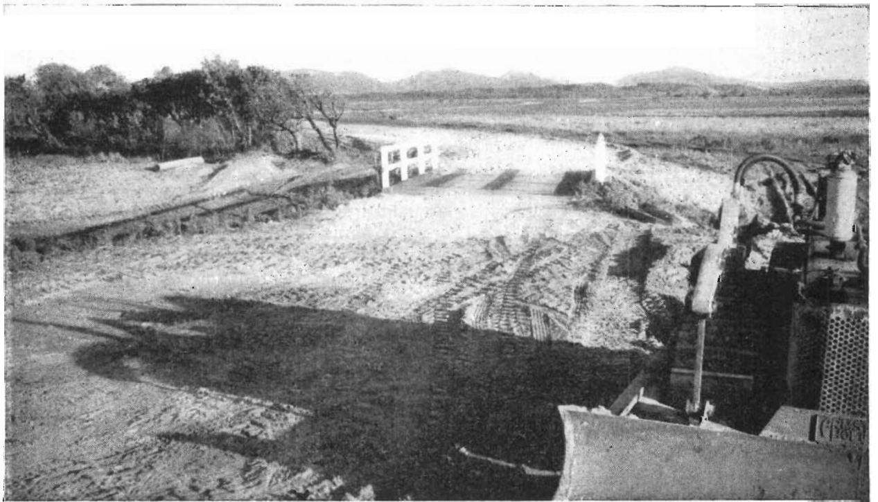
Plate 28.—Millar's Road in Yanakie Soldier Settlement Estate, South Gippsland Shire. Place 29.—Bridge on Millar's Road over outlet drain from Red Swamp, Yanakie Soldier Settlement Estate.
