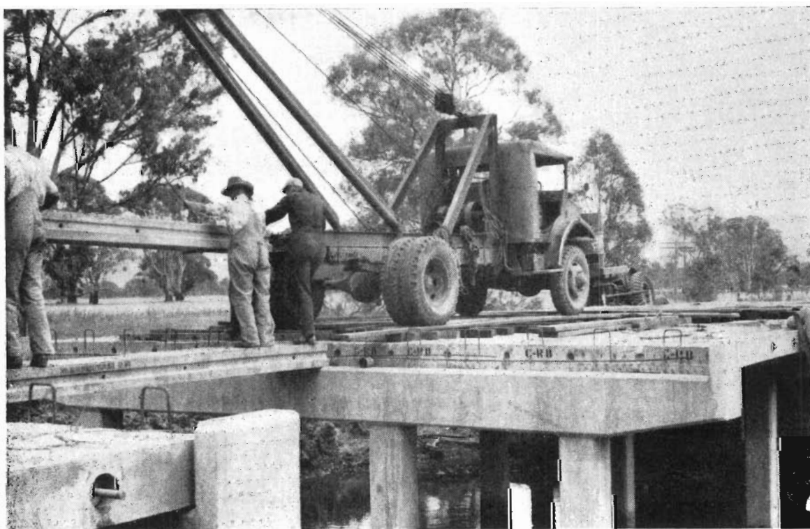
Plate 2.—Placing of 20-ft. prestressed concrete slab deck on bridge over Mt. William Creek at Mokepilly on Grampians tourists' road.
