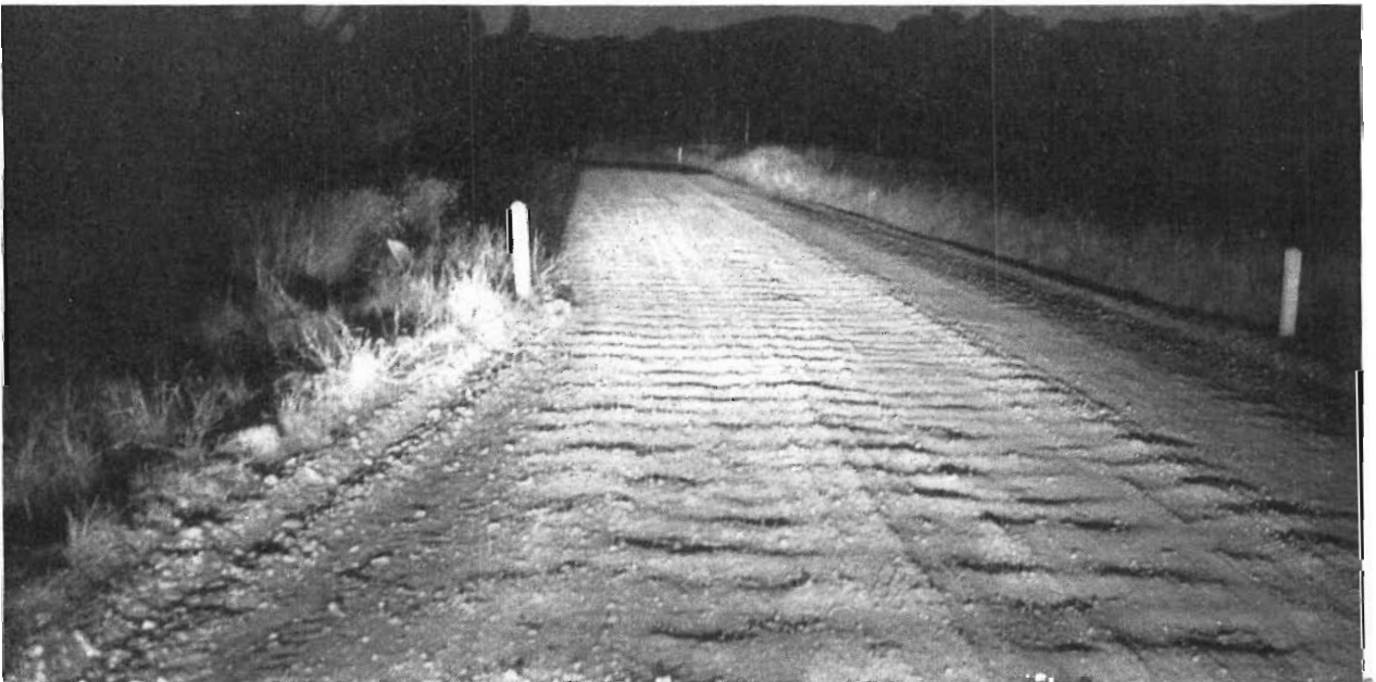
Plate 2.—Corrugated section of State Highway carrying 300 vehicles per day. Reconstruction and sealing delayed by lack of funds.
