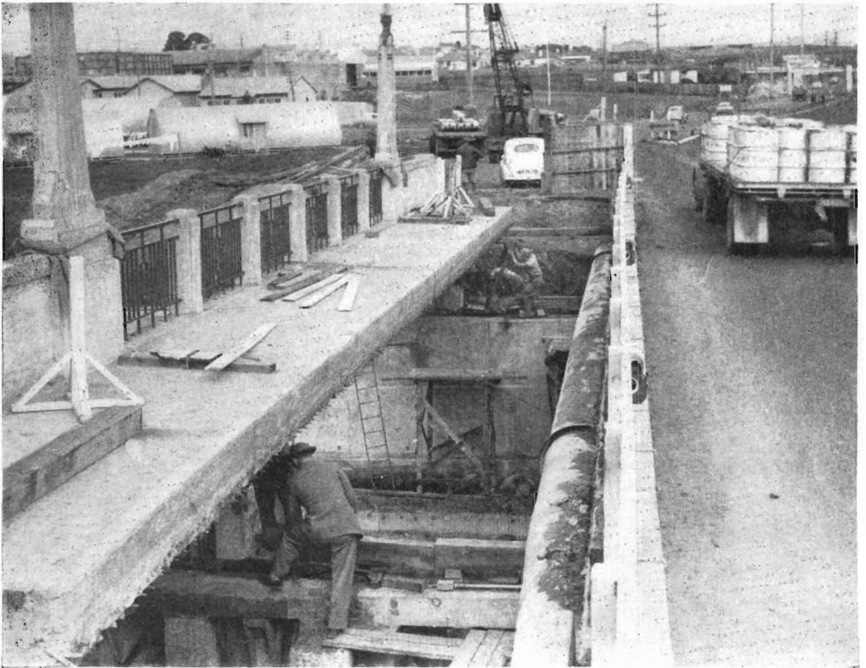
Plate 24.—Widening bridge over Gardiner's Creek, Warrigal Road, by jacking over handrails and footway.
