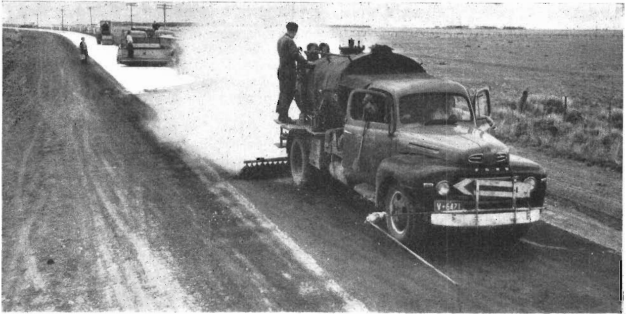
Plate 36.—Sealing work being carried out on the Rokewood Road at Shelford between Geelong and Rokewood. Shire of Leigh.
