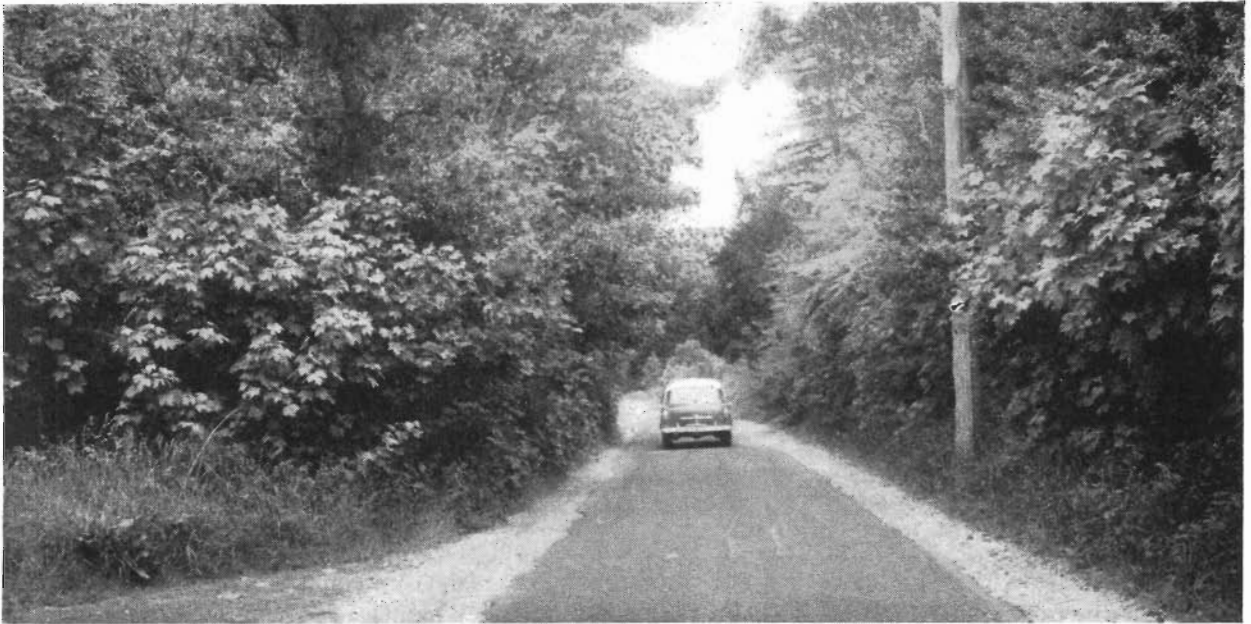
Plate 7.—Gisborne Shire—Mt. Macedon Road. Old narrow section one mile south of Camels Hump before reconstruction.
