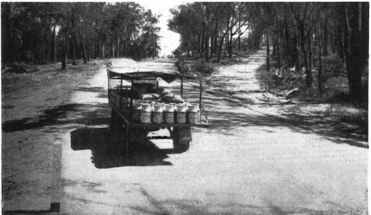
Plate 6.—Reconstructed hilly section Yarram-Traralgon Road near Carrajung Lower, showing old alignment on right.
