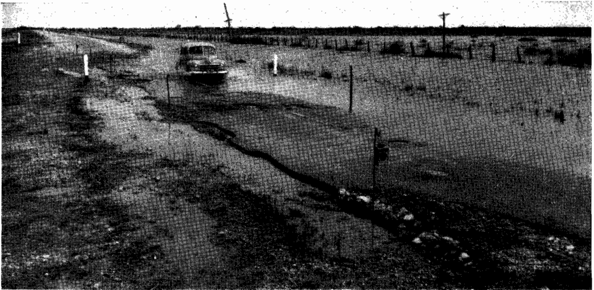
Plate No. 40.—The failed seal on the Loddon Valley Highway at 71 miles after flooding.
