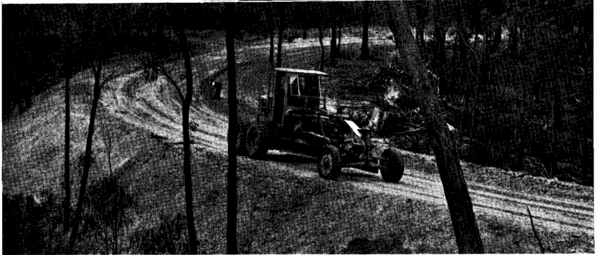
Plate No. 26.—Realignment and reconstruction in progress on the Walhalla Road between Gooding and Gould.
