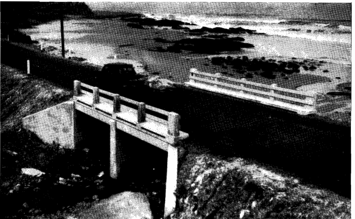
Plate No. 23.—New culvert over Stony Creek on the Ocean Road east of Lorne.
