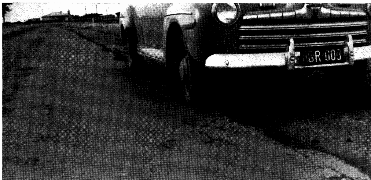
Plate No. 19.—Section of Princes Highway West 3 miles west of Colac before widening and resheeting.
