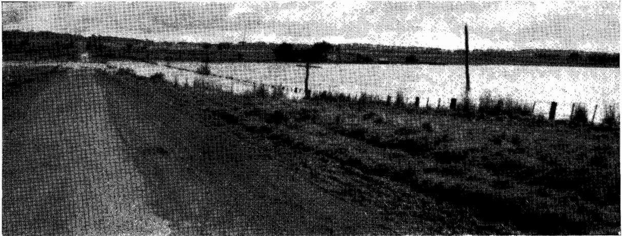
Plate No. 41.—Section of Midland Highway east of Corop which failed after flooding.
