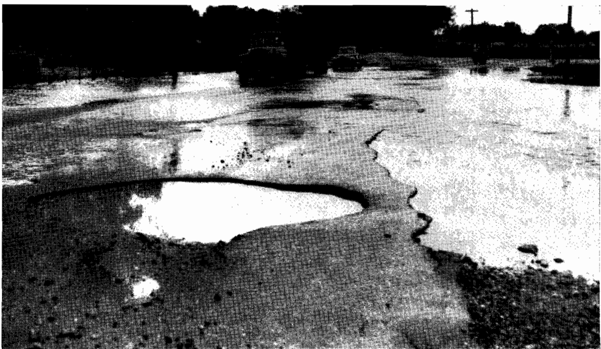
Plate No. 42.—Typical failures on the Hume Highway north of Wangaratta after flooding from the Ovens River.
