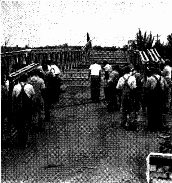
Plates Nos. 33 and 34.—A "Bailey" bridge was placed across the gap of 130 feet.
