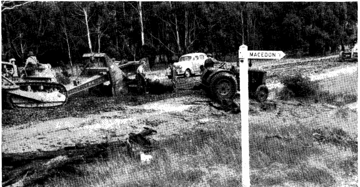
Plate No. 24.—Calder Highway, south of Woodend, showing removal of old corduroy base during reconstruction.
