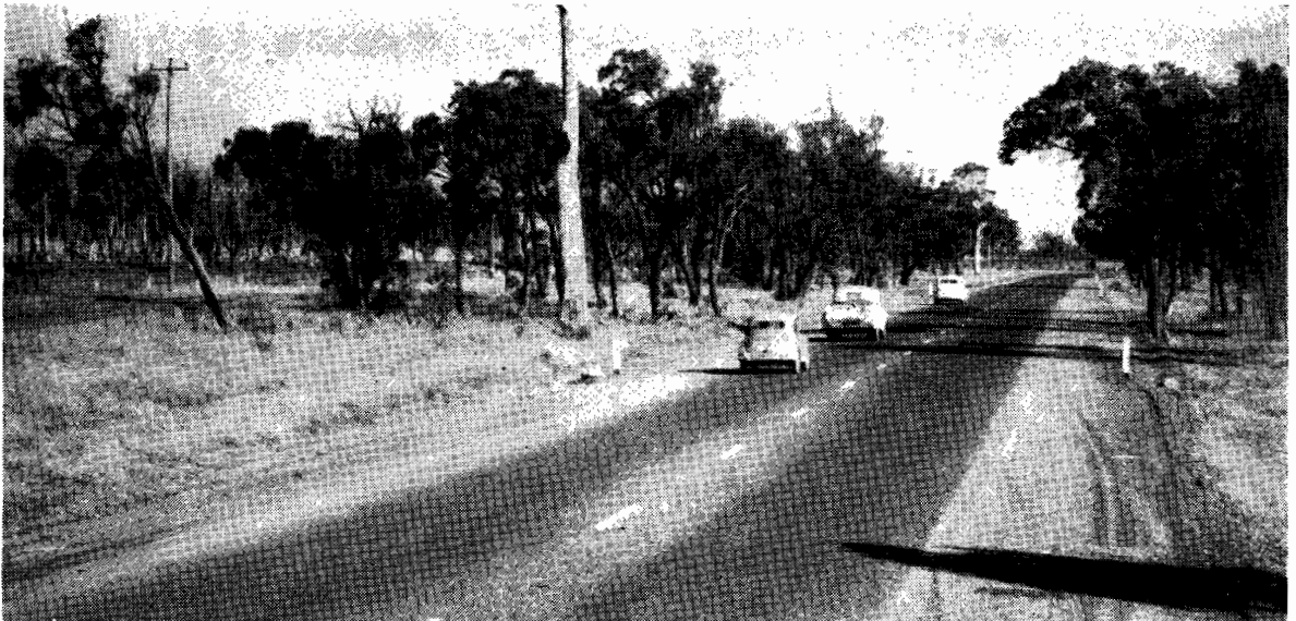
Plate No. 27.—A reconstructed section of the Princes Highway East, east of Morwell.
