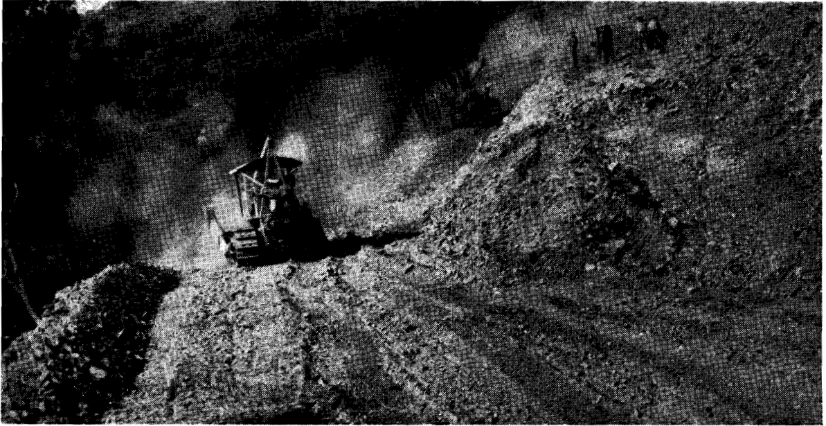
Plate No. 61.—Bulldozers working on reconstruction of Mansfield-Wood's Point Road north of Jamieson.
