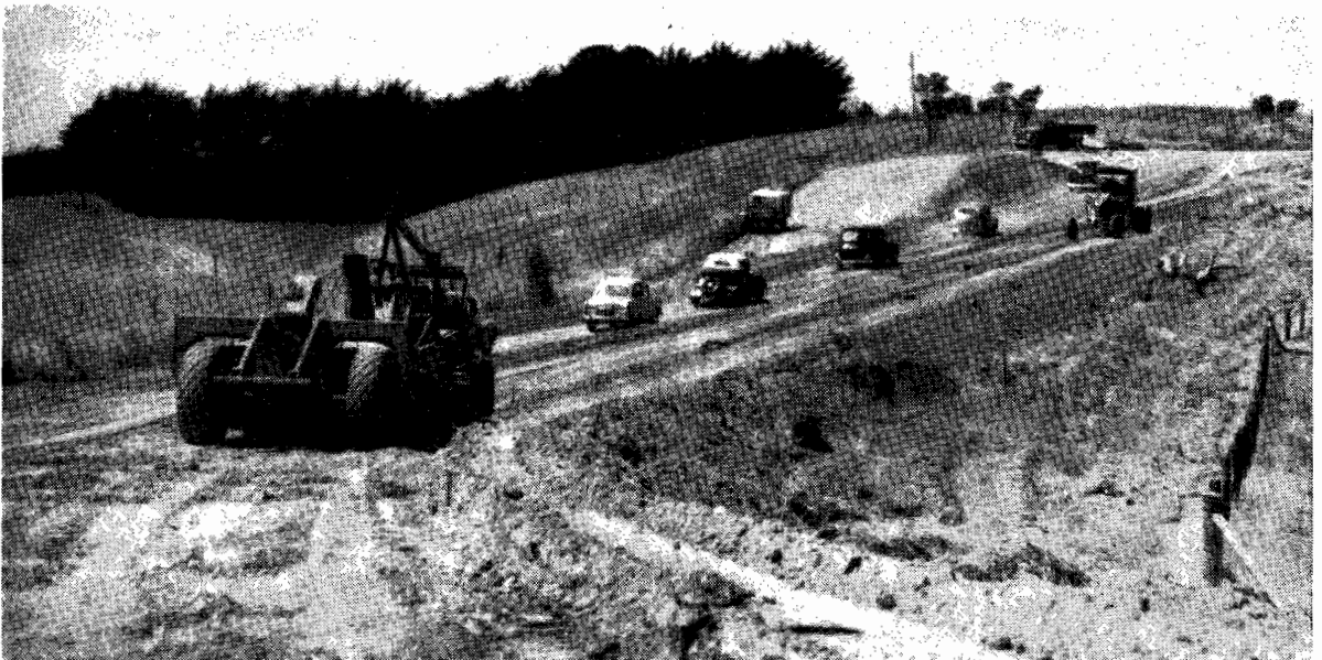
Plates Nos. 15 and 16.—Re-alignment and reconstruction of South Gippsland Highway, near Loch. Top plate shows old, narrow, rough road leading to sharp right-angled bend which has been eliminated.
