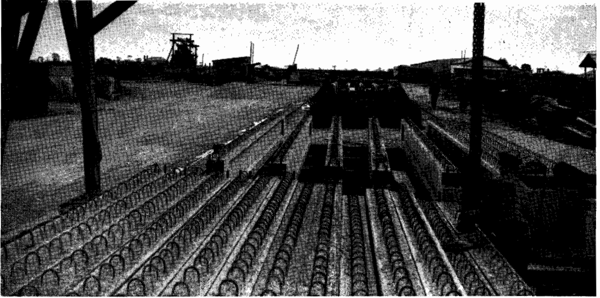
Plate No. 64.—Pre-cast beams in Bairnsdale Casting Yard, to be used on new bridge over Mitchell River.
