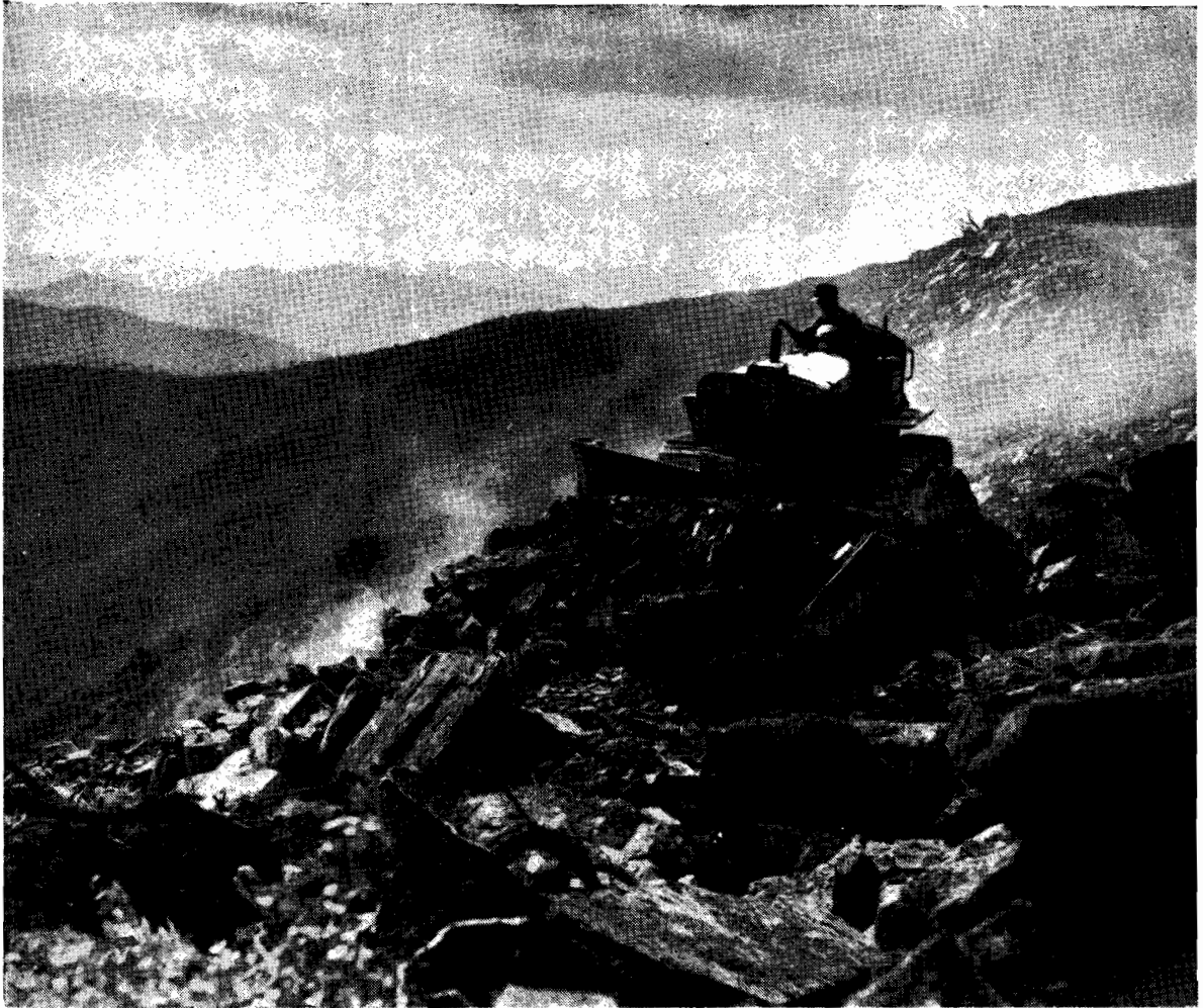
Plate No. 29.—Bulldozer at work on widening of the Alpine Road near Blowhard, Mt. Hotham.
