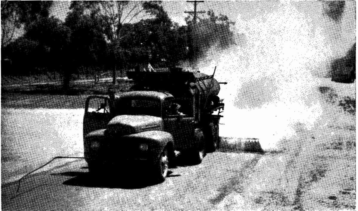
Plate No. 14.—Sealing in progress with 800-gallon sprayer on Murray Valley Highway at Nathalia.
