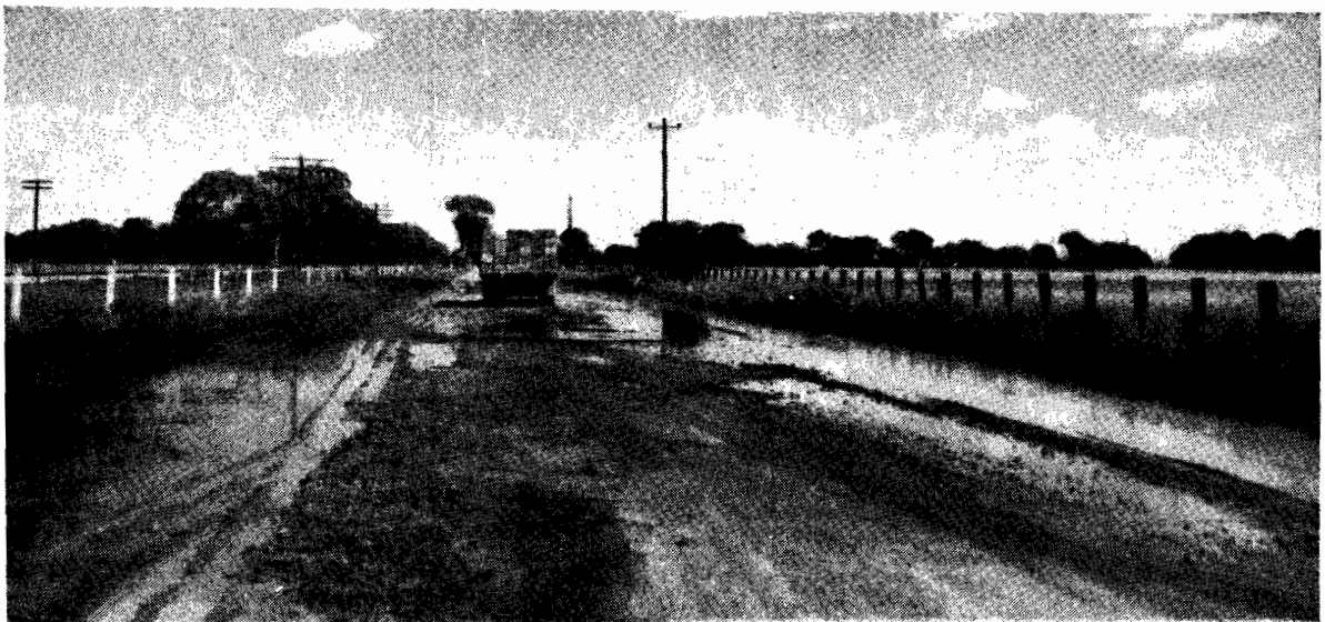
Plate No. 56.—Goulburn Valley Highway, approximately 124 miles, showing damage caused by floods.
