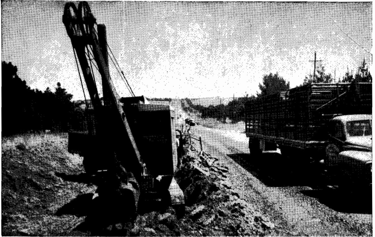
Plate No. 20.—Princes Highway East, approximately 25 miles, showing widening and regrading of vertical curve during reconstruction.
