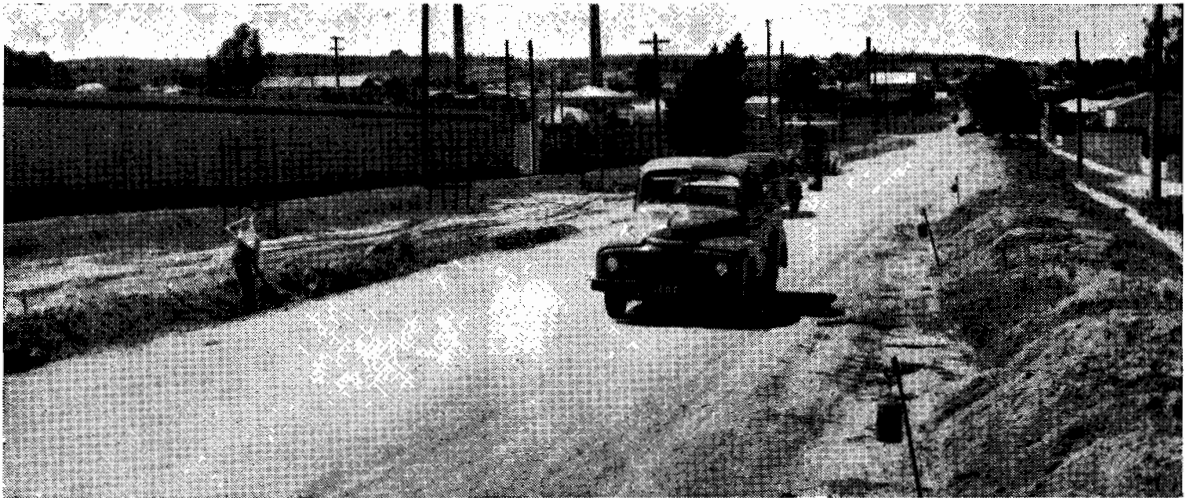
Plate No. 12.—North-Western Highway, near junction with Creswick Road, Ballarat, showing reconstruction in progress.
