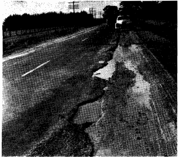
Plate No. 2.—Broken edges of seal on South Gippsland Highway.
