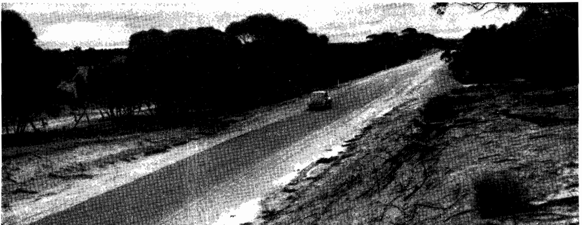
Plate No. 25.—Henty Highway at approximately 222 miles. Section reconstructed and sealed north of Hopetown.
