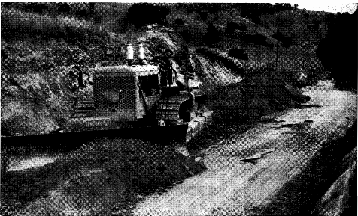
Plate No. 13. —Reconstruction and re-alignment of Murray Valley Highway at Bolga showing plant working.
