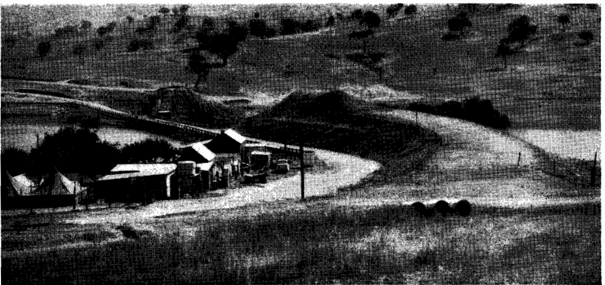
Plate No. 63.—New alignment and bank for Murray Valley Highway at Koetong Creek made necessary by the raising of the Hume Weir.
