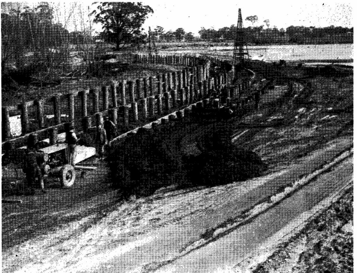
Plate No. 41.—Flood Protection Work in Progress on Marlo Road at Gilbert's Gulch, viewed from Marlo end.
