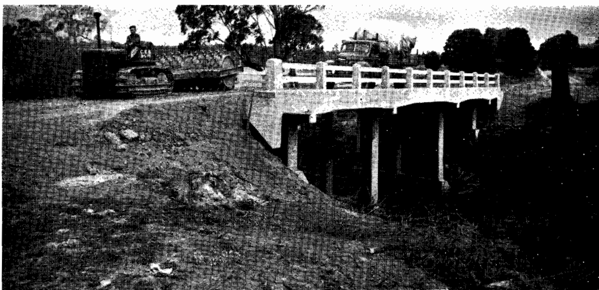
Plate No. 25.—Sheepsfoot Roller Consolidating Approaches to New Bridge over Morwell River on the Morwell-Mirboo Road.
