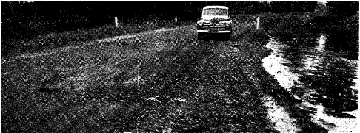
Plate No. 8.—Apsley Road seven miles north of Harrow where the high swamp level has ruined the road surface.
