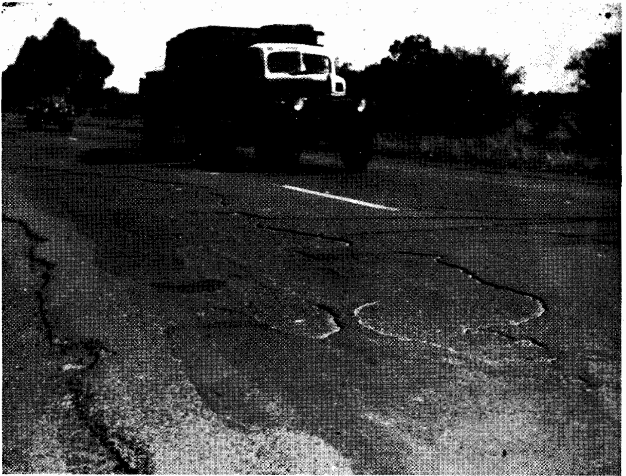
Plate No. 14.—Deteriorated Condition of Hume Highway North of Fawkner in 1951.
