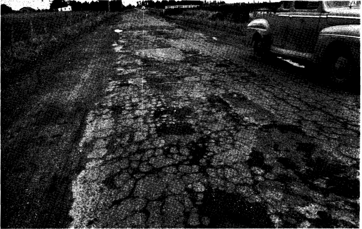
Plate No. 7.—A Badly Deteriorated Section of the Koo-wee-rup-Pakenham Road, three miles north of Koo-wee-rup.
