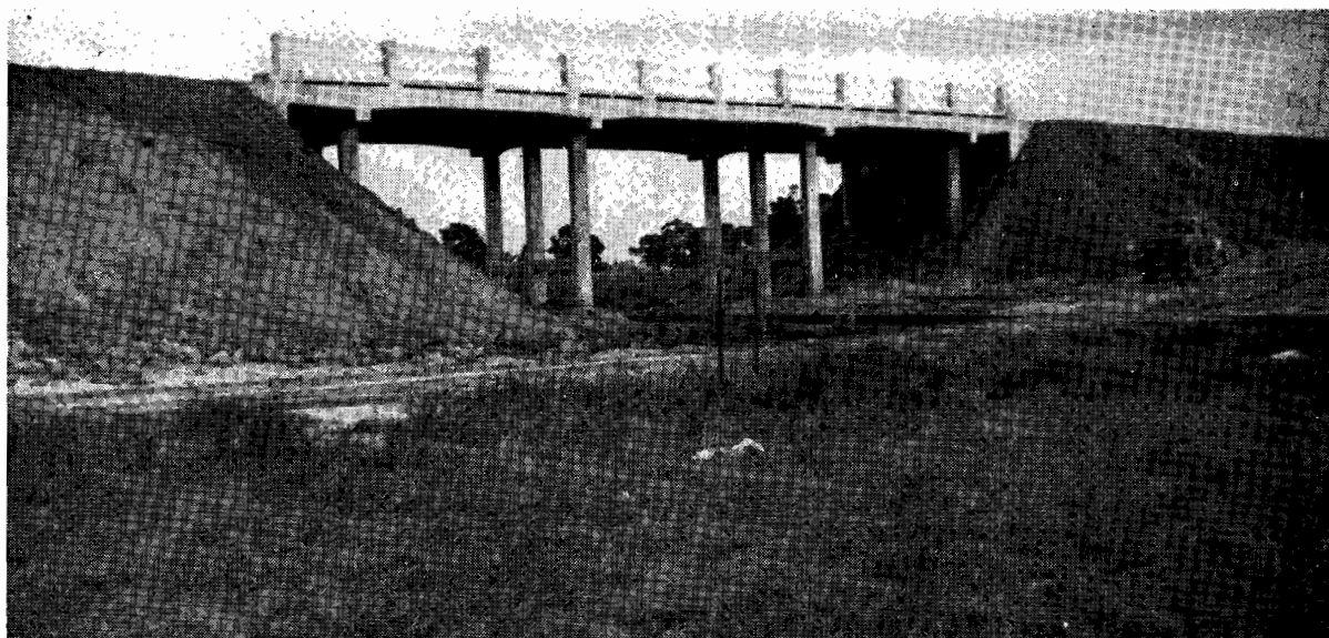
Plate No. 26.—Bridge on the Morwell-Maryvale Road over Railway Line to the Australian Paper Mills at Maryvale.
