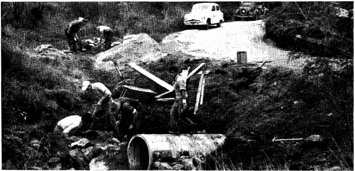
Plate No. 54.—A culvert constructed by voluntary labour on the Longwood-Ruffy Road.
