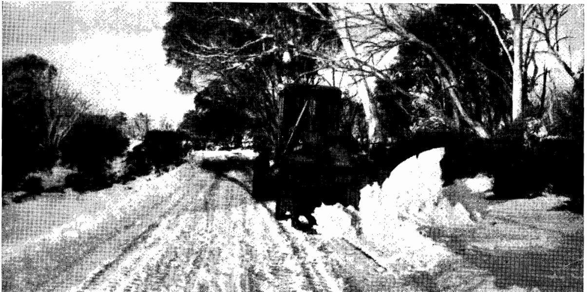
Plate No. 22.—Aveling Austin grader snow plough working on Alpine Road at Dinner Plain.
