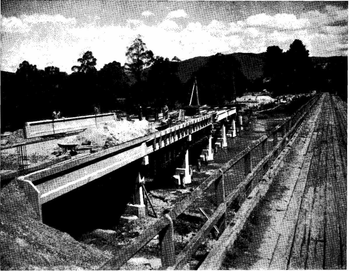
Plate No. 44.—New bridge under construction, and old bridge on Upper Goulburn Road over Goulburn River, near Thornton.
