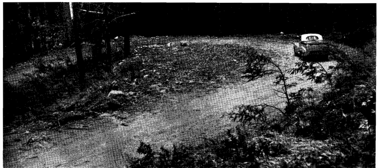
Plate No. 22.—Mt. Buller Road. Visibility improved by removal of bank at hairpin bend.
