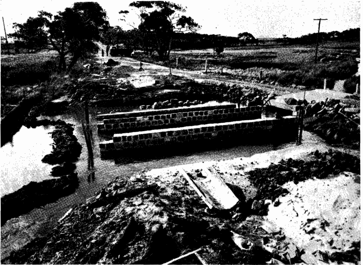
Plate No. 10.—Barrabool Shire : Anglesea Road. Reconstruction and enlargement of old inadequate culvert at Merrigig Creek.
