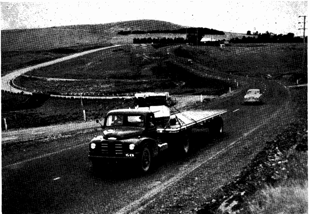
Plate No. 19.—Calder Highway. Reconstruction replacing old "Corkscrew" section, the scene of many serious accidents and fatalities.
