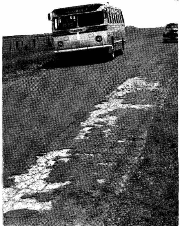
Plate No. 3.—Princes Highway West 195-200 miles, failed section West of Yambuk.
