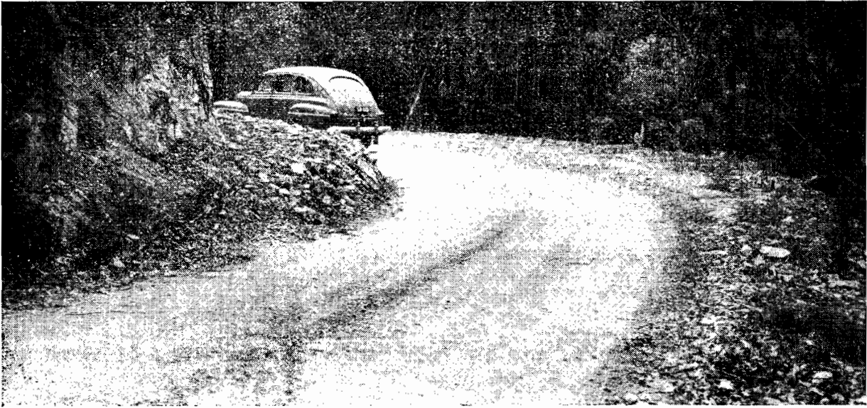
Plate No. 21.—Typical benching and widening on narrow side cutting of Walhalla Road (Forest Road) near Walhalla. Note benching for visibility.
