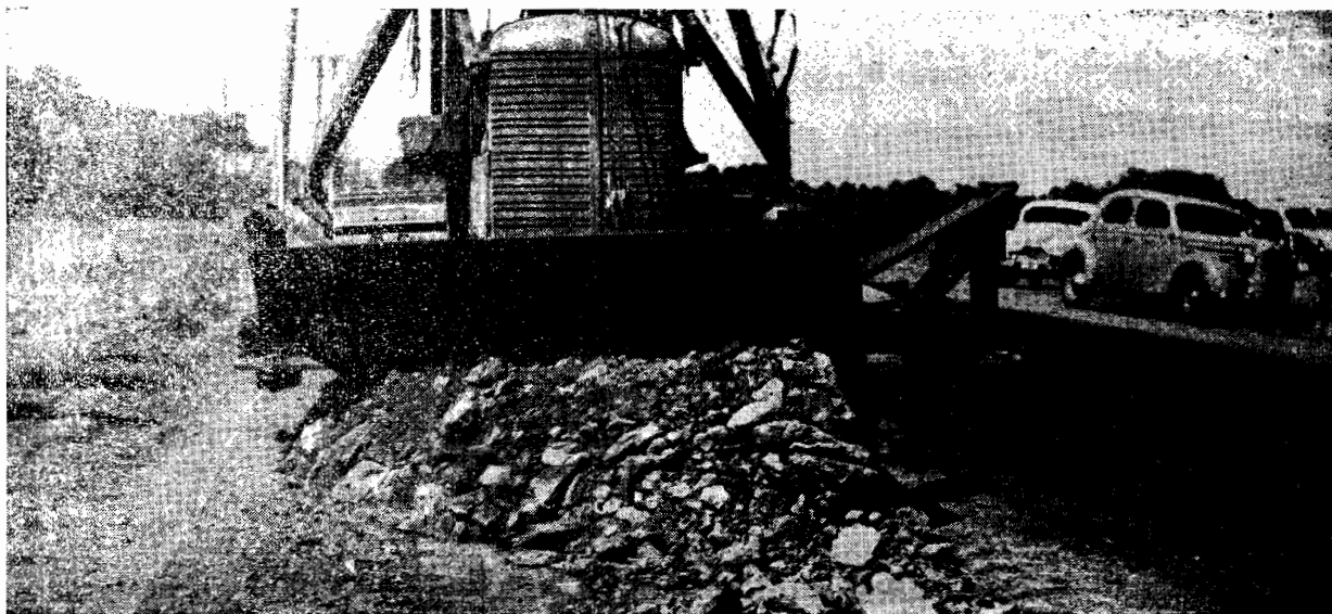
Plate No. 7.—A Trench Digging Attachment on a Bulldozer in use on the widening of the Hume Highway near Campbellfield. In one operation this apparatus excavates a trench of the correct depth and width.
