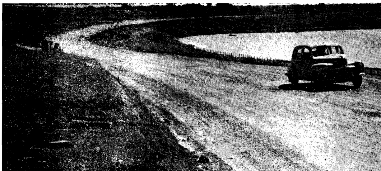
Plate No. 16.—A section of the North-Western Highway at Swanwater which has been entirely reconstructed, strengthened and widened after extensive failures.
