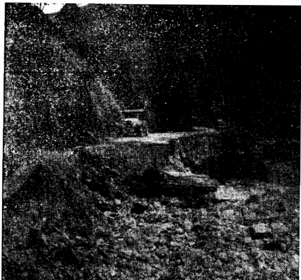
Plate No. 25.—The road was completely washed out at this section.
