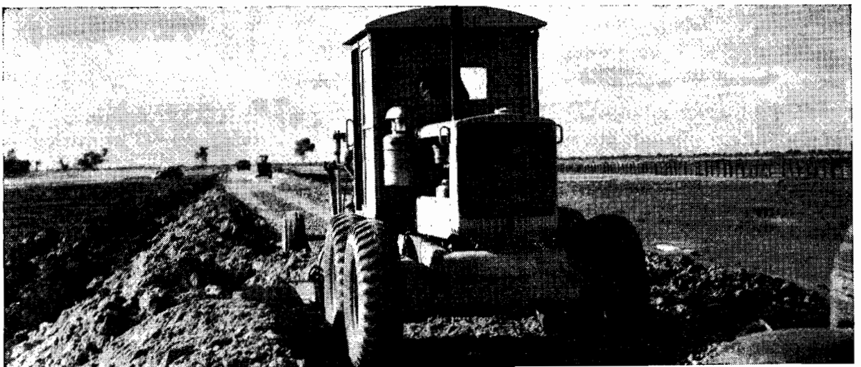
Plate No. 50.—A heavy grader at work on the same section of the Loddon Valley Highway.
