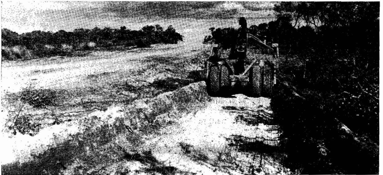
Plate No. 2.—A Heavy Tractor and Scoop working on the Hattah Deviation on the Calder Highway, south of Mildura. This Deviation will replace an old, rough tortuous track, and will shorten the Calder Highway by six miles.
