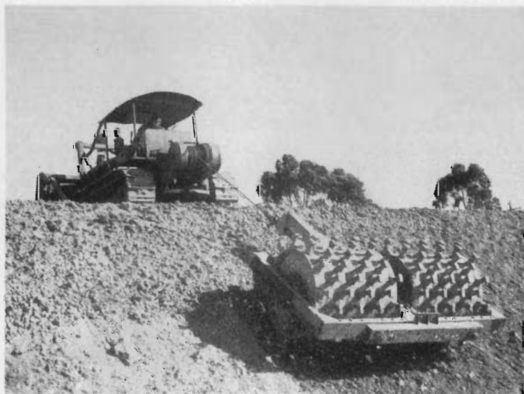
33. Princes Highway East. Consolidation of batter in filling by sheep's foot roller controlled by logging winch.
