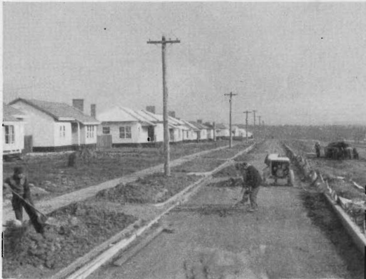
32. Princes Highway East. Service road in course of construction along route of proposed new highway south of Moe.
