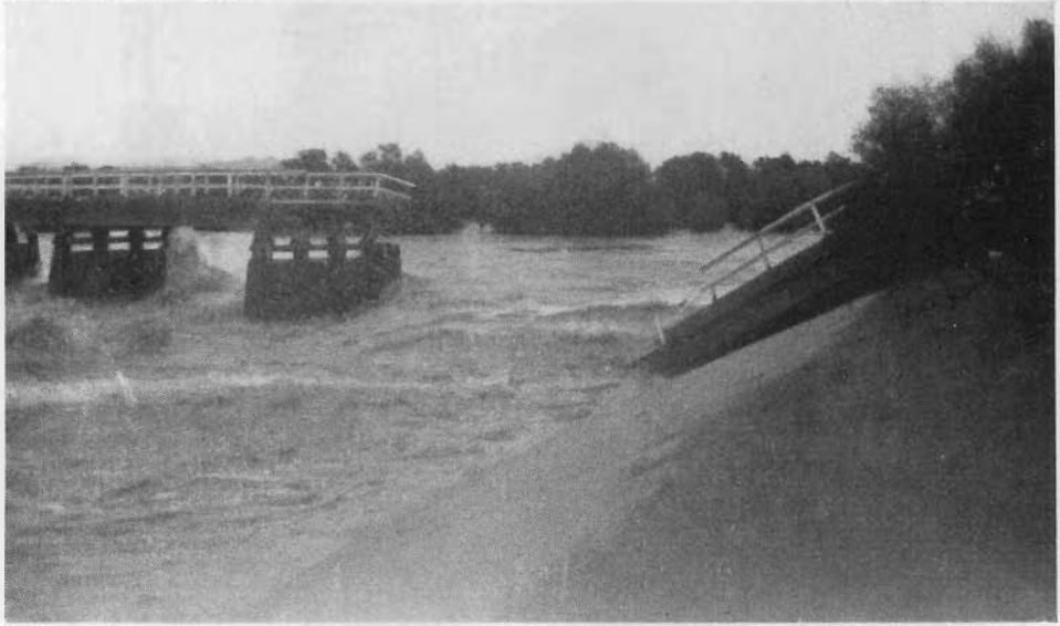
14. Princes Highway East, showing collapsed spans of bridge over Avon River at Stratford.
