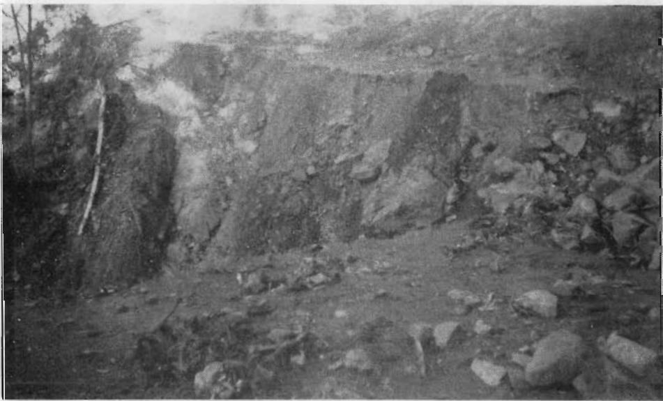
22. Suggan Buggan Road (East Gippsland). General view of washaway.
