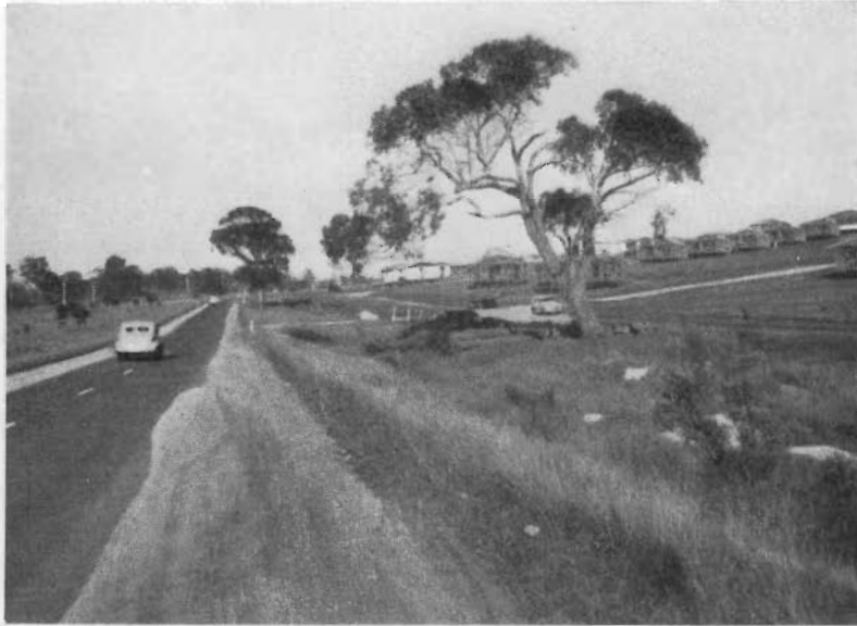
31. Princes Highway East near Morwell. Showing houses in course of erection by Housing Commission and roads being constructed by Board. Subdivisional road has been provided inside Estate and parallel with highway.
