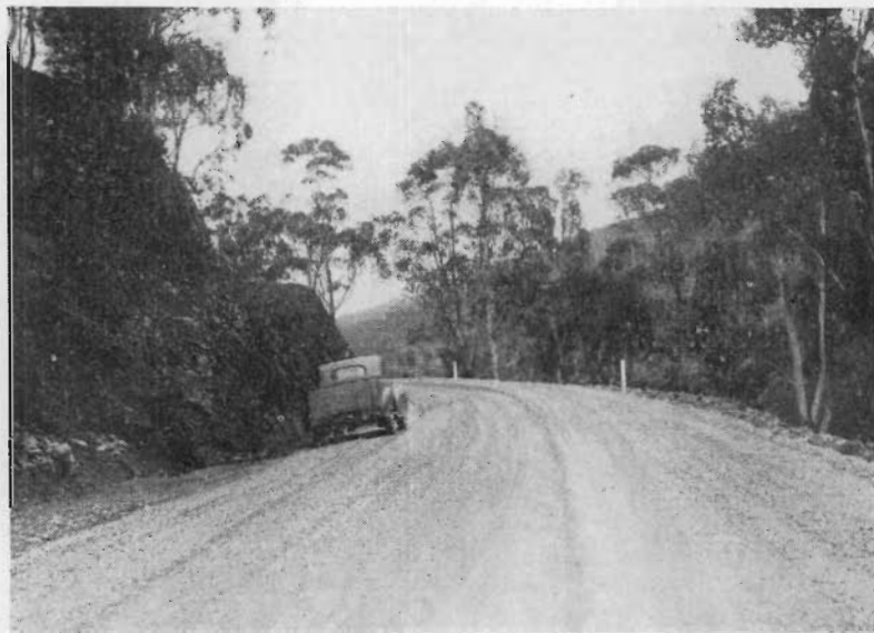
35. Kiewa Valley Road. Hilly section completed with crushed rock surfacing prior to sealing.
