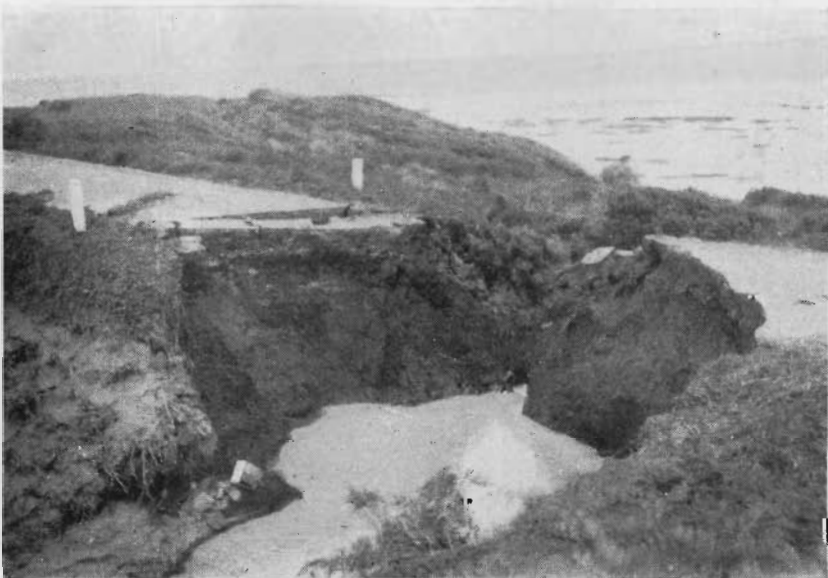
28. Ocean Road. Washaway at Chapman's Creek—October, 1949.
