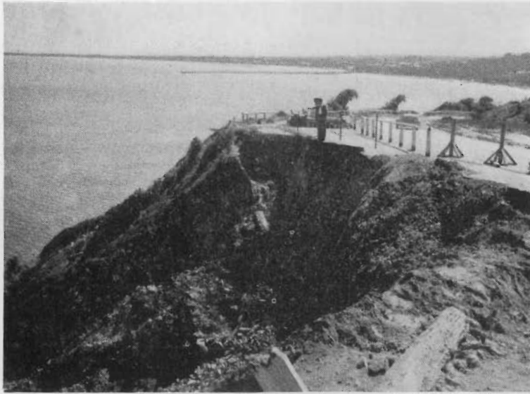
1. Nepean Highway. Subsidence at Oliver's Hill, Frankston.
