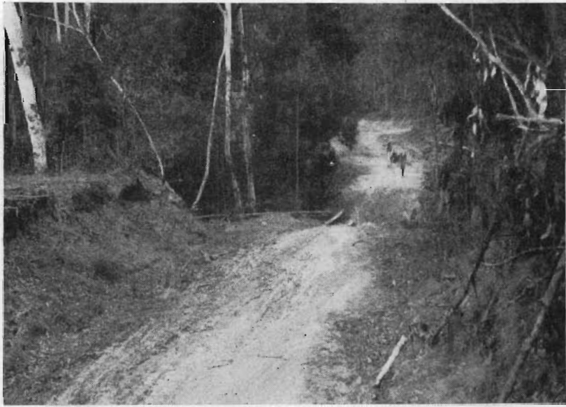
7. Lockhart's Gap Road. General view of old road showing burnt out culvert.
