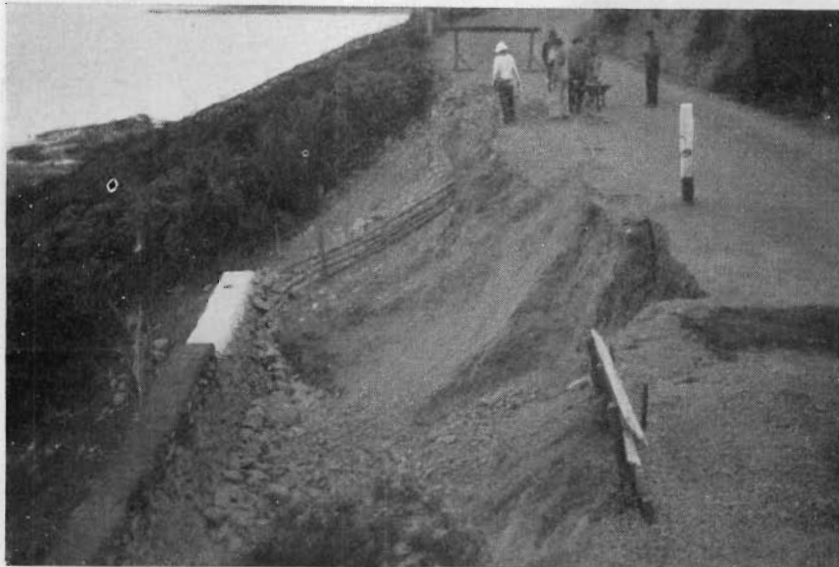
29. Ocean Road. Typical damage to outside edge of road, and retaining wall in course of construction.
