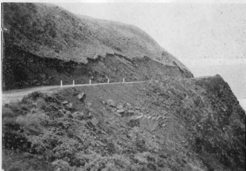
30. Ocean Road. Retaining wall built following landslip near Cape Patten in November, 1949.
