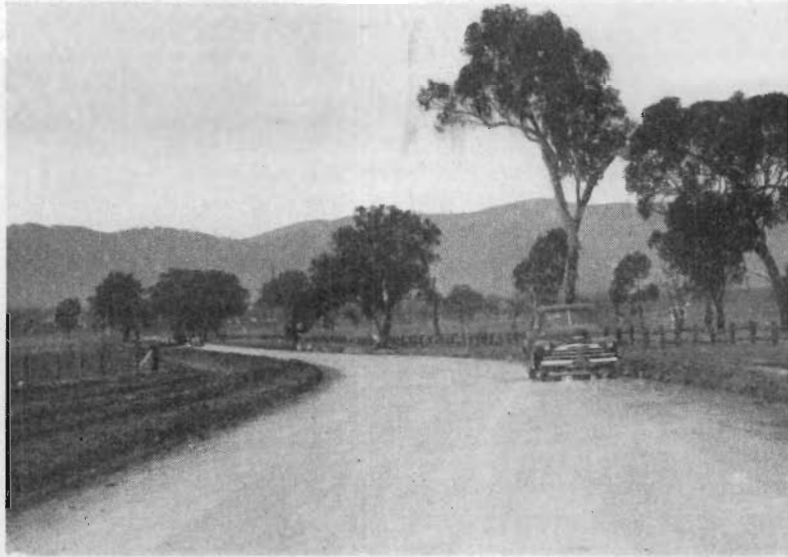
34. Kiewa Valley Road. Deviation constructed and base course of consolidated river gravel laid.
