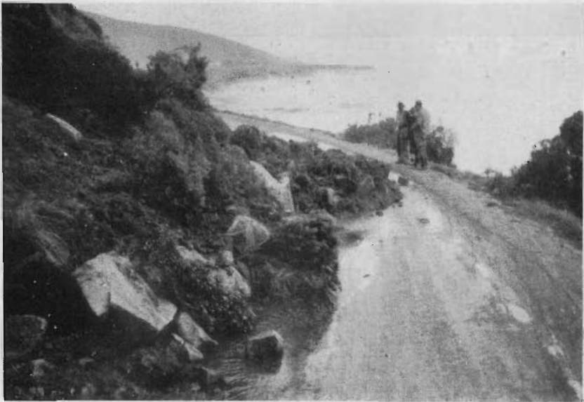
27. Ocean Road. Typical land slip following flood—October, 1949.
