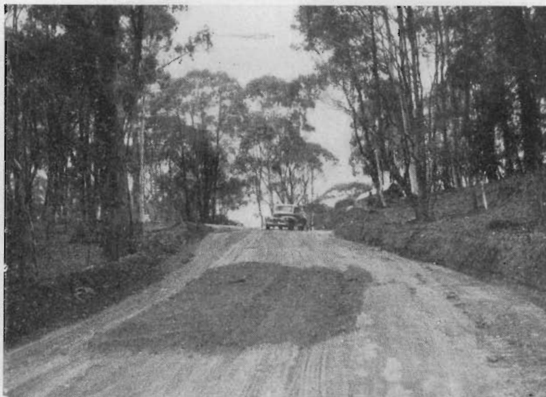
9. Lockhart's Gap Road. Road on saddle of Gap after reconstruction. Spreading granitic sand is in progress.
