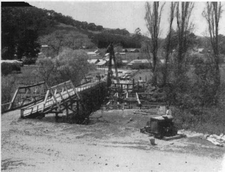
Plate No. 5. Old timber bridge over Jamieson River at Jamieson. New bridge in course of construction.
