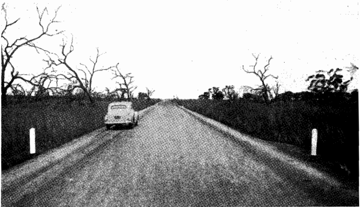
Plate No. 10.—Murray Valley Highway. Newly-sealed sand-clay pavement at Murphy's Swamp, 10·8 miles north-west of Echuca.
