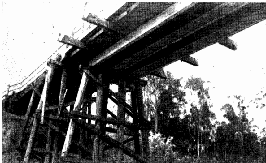
Plates Nos. 18 and 19.—Princes Highway East. Bridge over Boggy Creek at Nowa Nowa. Showing joists and new supporting piers.
