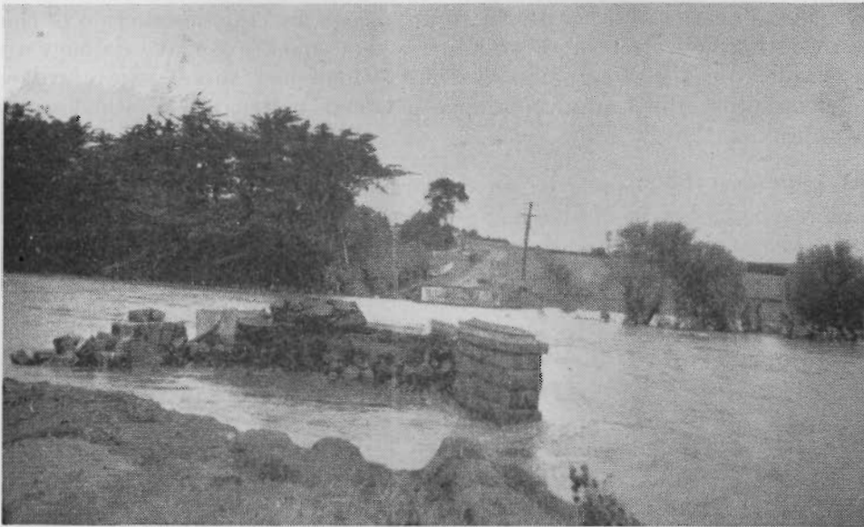
PLATE 12.—Warrnambool—Caramut Road—site of Cassidy's bridge destroyed by flood.
