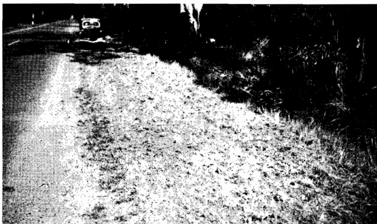
PLATE 8.—Princes Highway East, near 54 mile. Pavement margin after treatment with rotary hoe.
