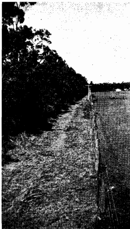
PLATE 7.—Princes Highway East, near 54 mile. Strip at road boundary after treatment with rotary hoe.
