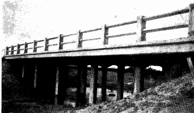
PLATE 1.—Dandenong Shire—Spring Vale Road.—Bridge over main drain (sheeting of embankment not completed).
