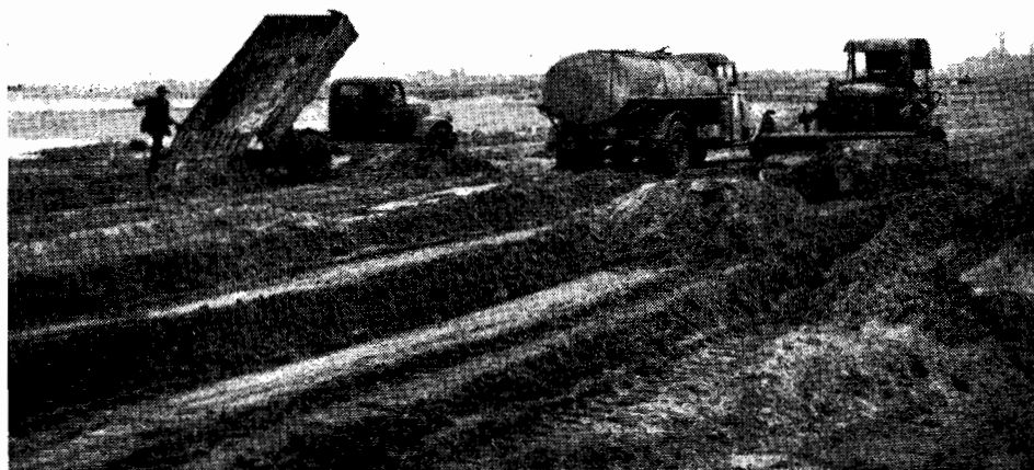
PLATE 27.—Spreading sand filling for construction of runways, Fisherman's Bend, and consolidation by watering and trafficking.
