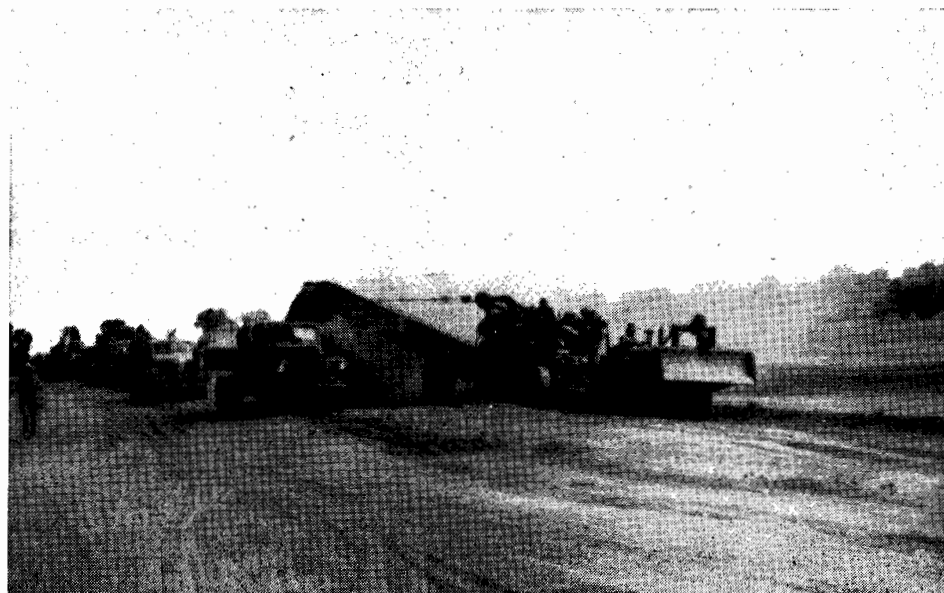
PLATE 21.—Winning limestone rubble with elevating grader, for strengthening section of Stuart Highway near Wycliffe prior to construction of bituminous surfacing.
