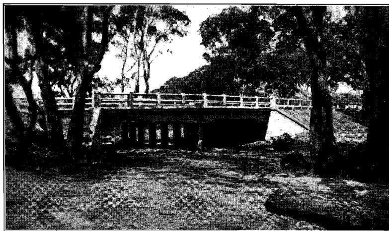
Plate No. 1.—Showing widened bridge over Castle Creek on the Hume Highway.
