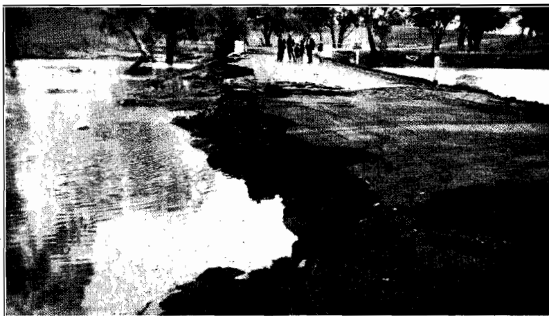
Plate No. 14.—Showing flood damage to Midland Highway at Nalinga.
