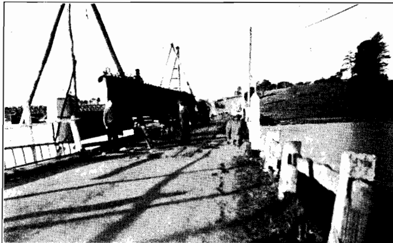
Plate No. 32.—Showing progress of work on the Nicholson River bridge to the 30th June, 1939.
