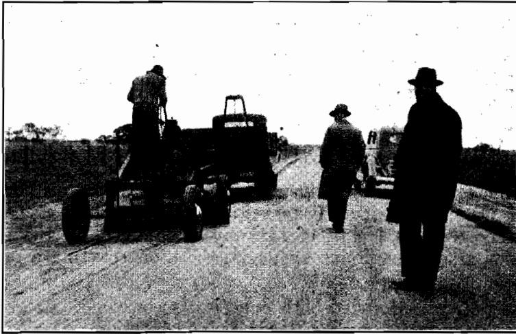
Plate No. 1.—Showing grader at work on shoulder of a section of the Murray Valley Highway.
