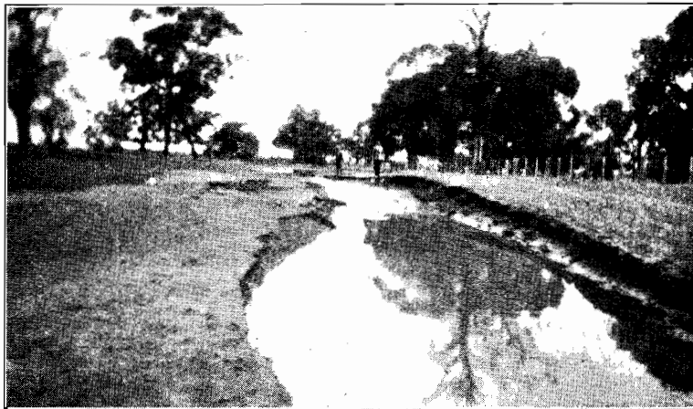
Plate No. 39.—Showing damage on the St. Arnaud Main Road in the Shire of Charlton.
