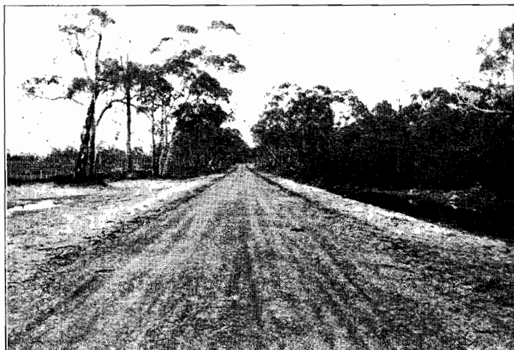
Plate No. 31.—Section of the Drik Drik-Nelson Road in the Shire of Portland, constructed from Unemployment Relief Funds.
