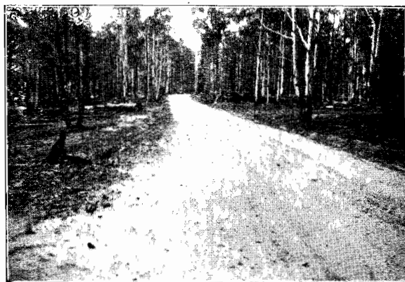
Plate No. 25.—Recently gravelled surface on Tolmie-Whitfield Road in the Shire of Oxley.
