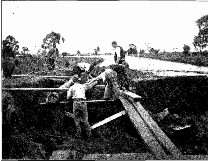
Plate No. 16A.—Another view showing damage by floods at bridge over the Bunyip River on the Prince's Highway.
