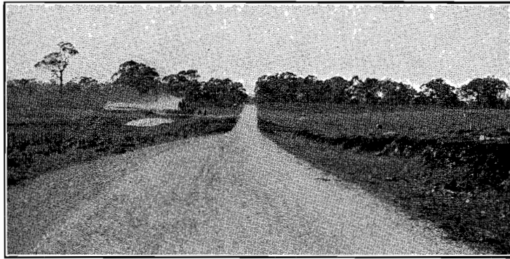
Plate No. 5.—Showing section of Prince's Highway between Dartmoor and South Australian Border preparatory to sealing.
