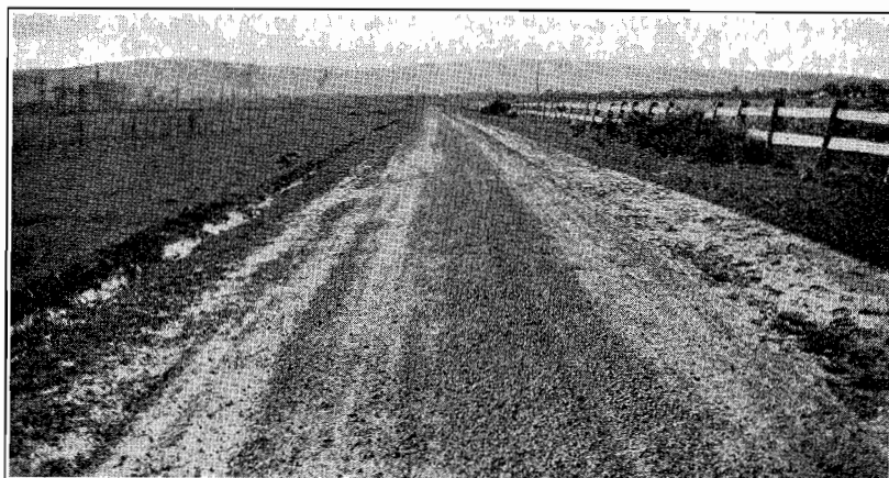
Plates Nos. 25 and 26.—Showing Rossiter's Road, South Gippsland, before and after partial construction.
