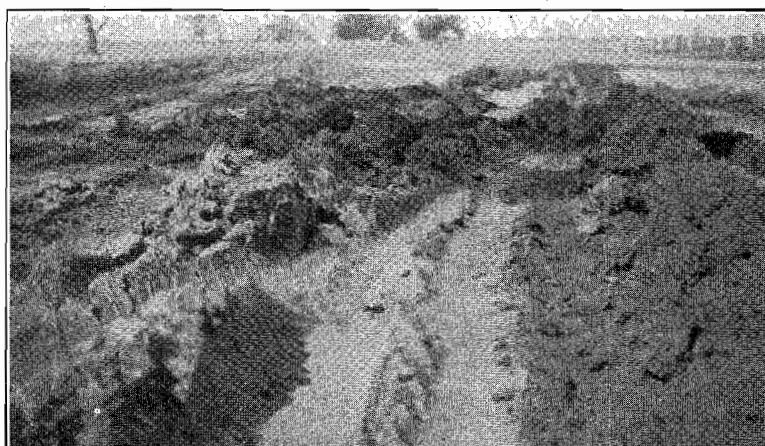
Plate No. 11.—Showing damage on Main Road, between Minyip and Warracknabeal, caused by excessive loads.
