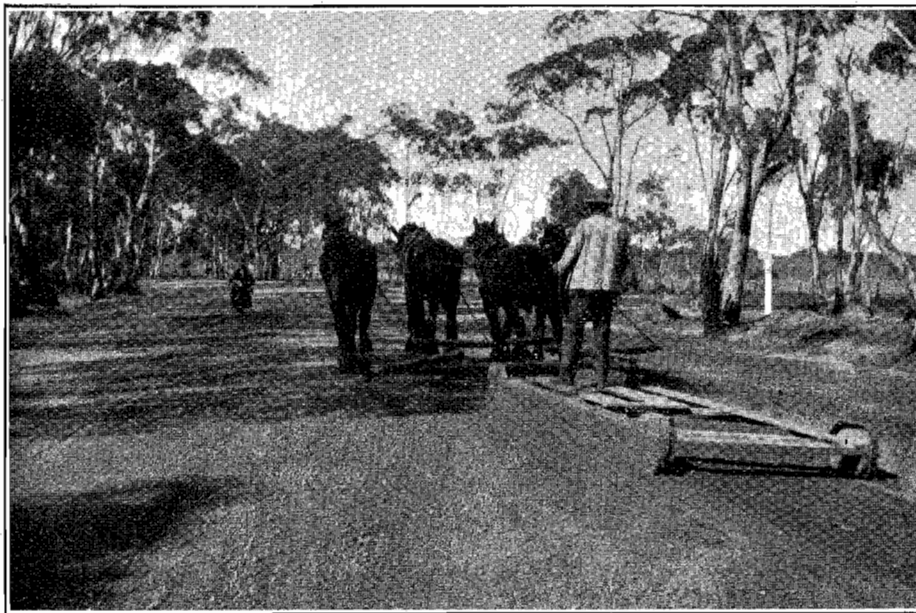
Plate No. 21. Maintenance of Gravel Road with Road Planer after Scarifying and Grading until Surface Sealing is carried out.
