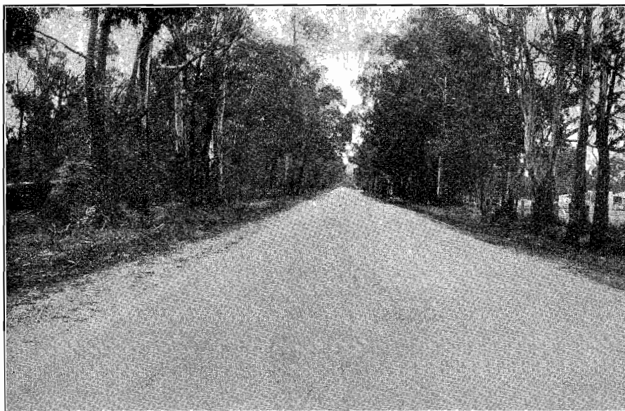
Plate No. 18.—Bituminous seal coat on granitic sand on the Prince's Highway East in Buln Buln Shire.
