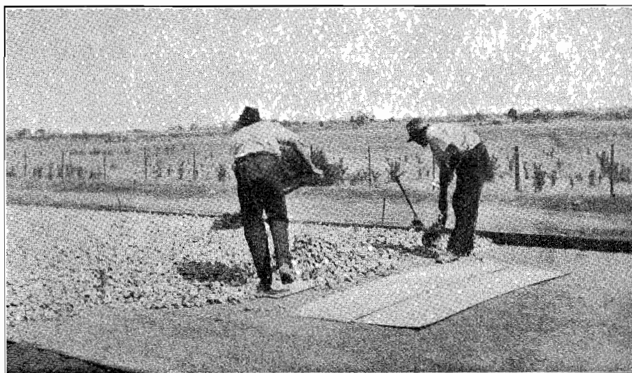
Plate No. 13.—Calder Highway. Spreading metal for bituminous macadam surfacing. Day labour works at Malmsbury.
