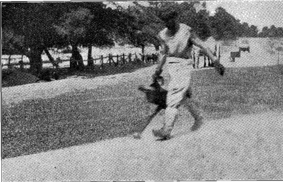
Plate No. 16.—Sealing bituminous macadam surfacing by hand. 3 gallon per square yard.
