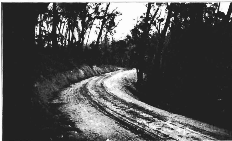
Plate 26. Showing grading and side-cutting at Haunted Hills, main Gippsland Road, Morwell Shire.
