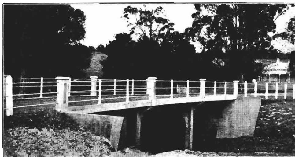
Plates 17 and 18. Showing the old and the new bridge, Bendigo Road, Chewton Borough.
