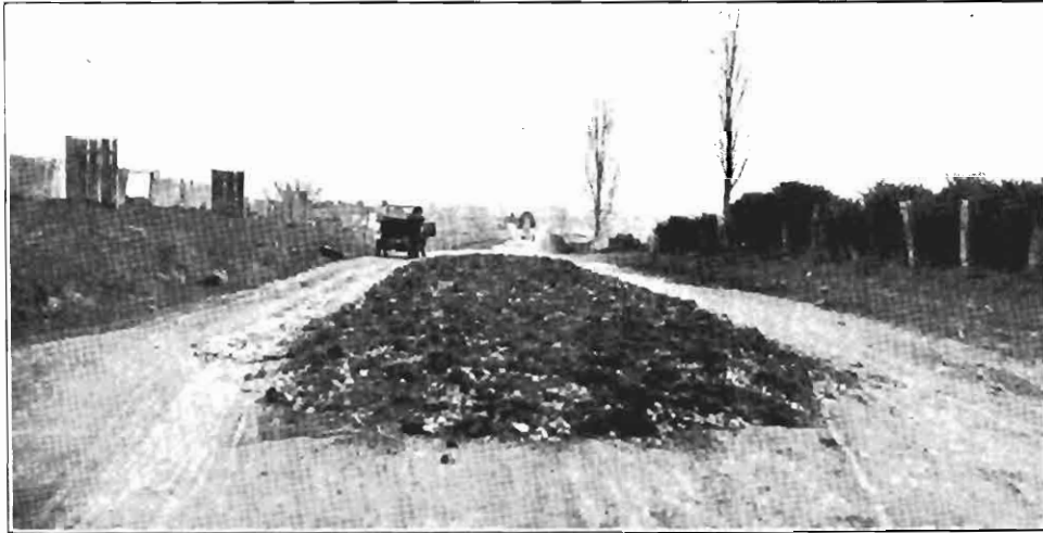
Plate 9. Showing improper and wasteful practice of binding repair metal with volcanic soil.
